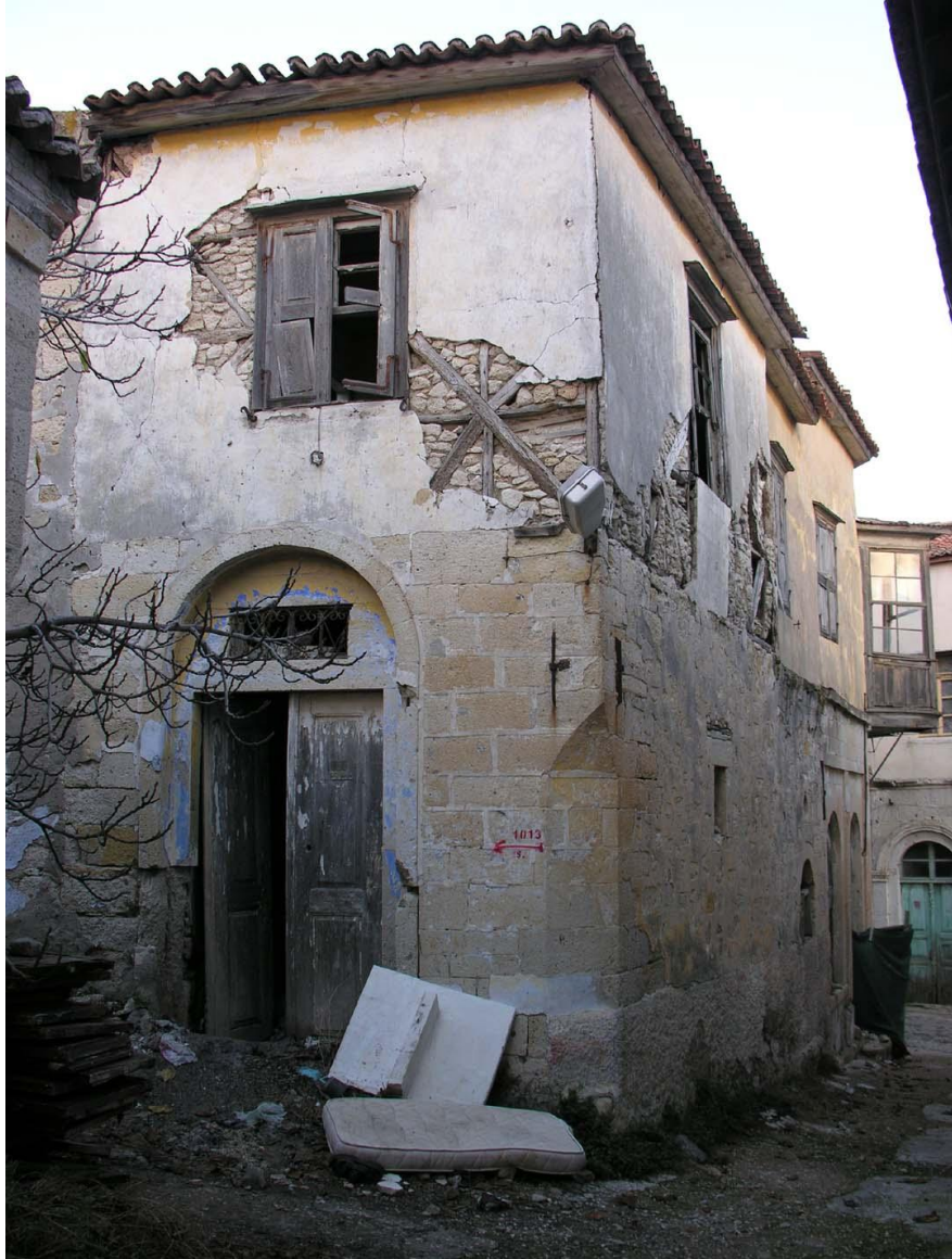
Figure 3.11. Hybrid construction (cut-stone masonry in first floor, wooden brace structure filled in between with rubble stones in the second floor walls, wooden roof with tiles (alaturka) on top, in Hacı Memiş Quartier)
