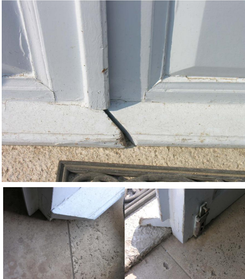
Figure 3.35. An example of door sash detail of an Alaçatı House (Taş House)
