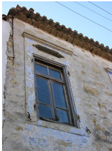
Figure 3.38. Example of NV opening detail (menfez) over a window from an Alaçatı House
