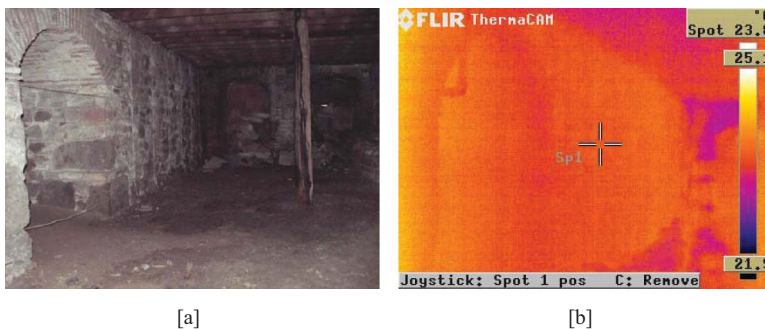
Figure 14. A) Photograph and B) infrared thermographic image of the wall #5 of the basement showing rising damp (September 23, 2005) (figure is provided in color online).
