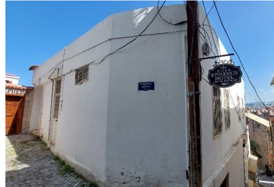
Condition Class 0: Housing (DRH2)
