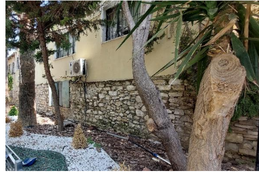
Condition Class 2: Fortification Wall (CRW5)
