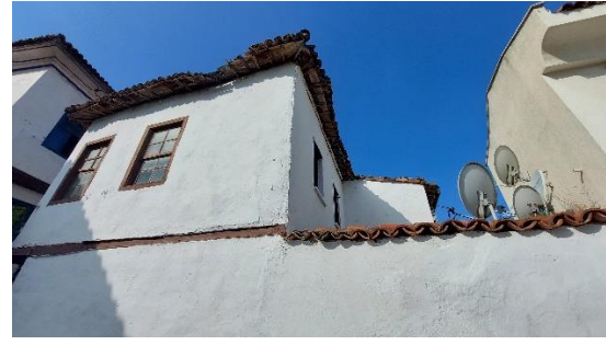
Condition Class 2: Housing (CRH4)
