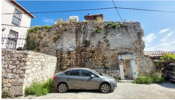
Condition Class 3: Fortification Wall (DRW2)
