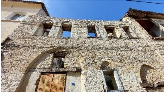
Condition Class 3: Housing (DRH5)
