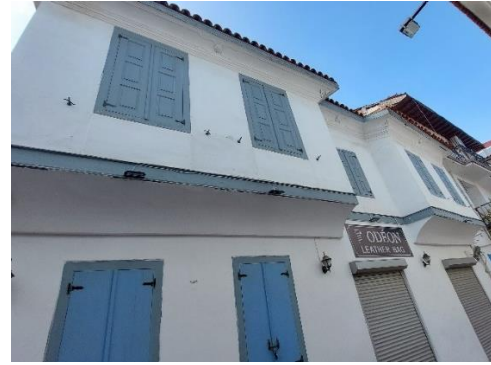
Condition Class 0: Housing (CRH5)
