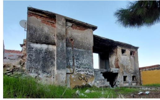
Condition Class 2: Housing (DRH14)
