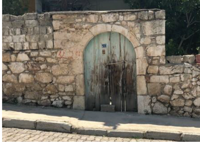
Figure 60. A courtyard gate in Kale constructed with the replaced building material (Source: Etlacakus and Turan 2019, 470).
