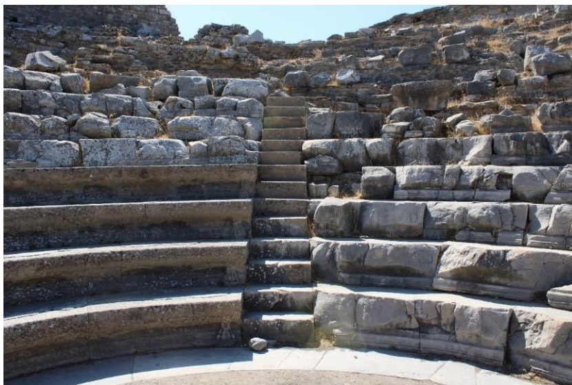
Figure 4.51. Completed seating rows and completed and reconstructed stairs by using concrete (Photograph: T. Tekin, 05.09.2021).
