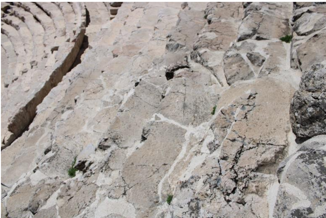
Figure 4.107. Completed seating rows in the north upper side of the cavea with mortar and original seating row remains (Photograph: T. Tekin, 09.04.2022).
