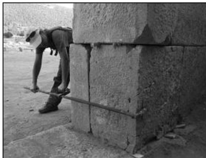
Figure 4.69. Reinforcement implementation in the cut stone blocks (Source: 28. Kazı Raporu, 1. Cilt, p.28 Figure:13, 2005)
