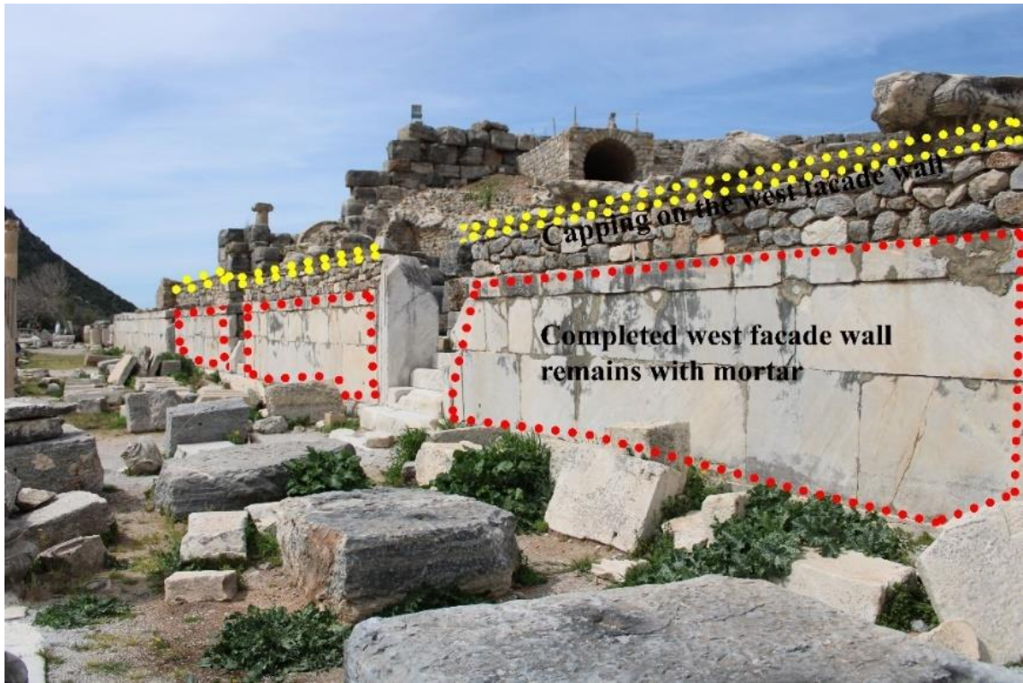
Figure 4.19. Interventions on the outer part of the south wall (Photograph: T. Tekin, 03.04.2022).
