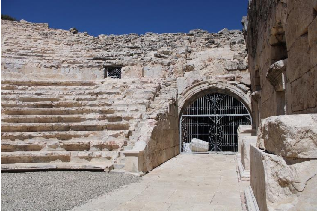
Figure 4.106. Completed seating rows with mortar in north side, partially reconstructed part at the beginning of the north analemma wall and completed pulpitum flooring with mortar (Photograph: T. Tekin, 09.04.2022).
