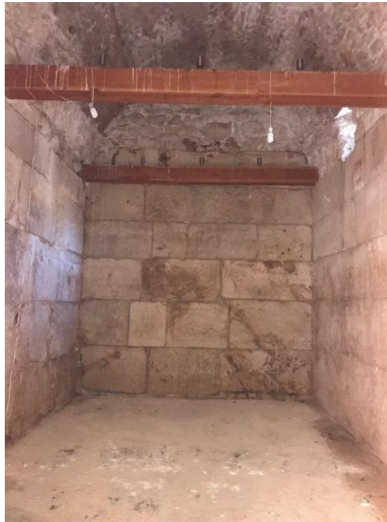
Figure 4.66. Wooden tensioners added to ensure the structural integrity of the walls made of cut stone blocks in the vaulted room on the northern direction (Photograph: T. Tekin, 08.04.2021).
