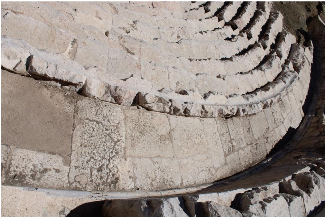
Figure 4.110. The completion of the stone gaps at the diazoma with mortar and partial reconstruction with concrete (Photograph: T. Tekin, 09.04.2022).
