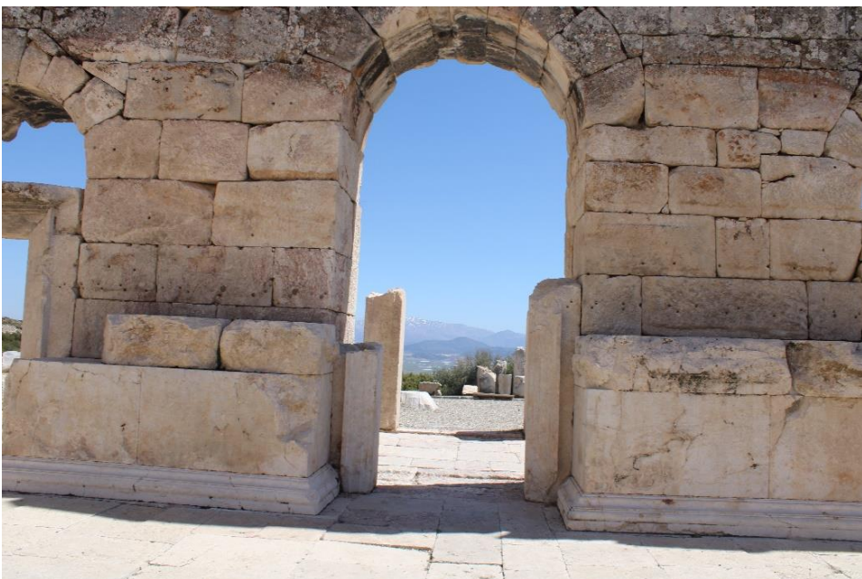
Figure 4.89. Traces of fastener remains on the west side of the scene wall (Photograph: T. Tekin, 09.04.2022).
