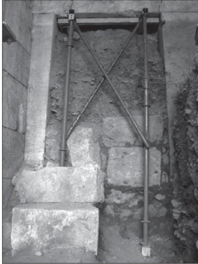
Figure 4.67. Static strengthening work at the north gate (Source: İşkan Işık 2011, p.21 Figure:25).
