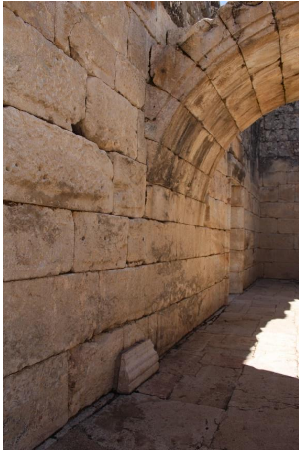
Figure 4.103. Fixing plinth-like remain to the south section of the scene wall with mortar (Photograph: T. Tekin, 09.04.2022).
