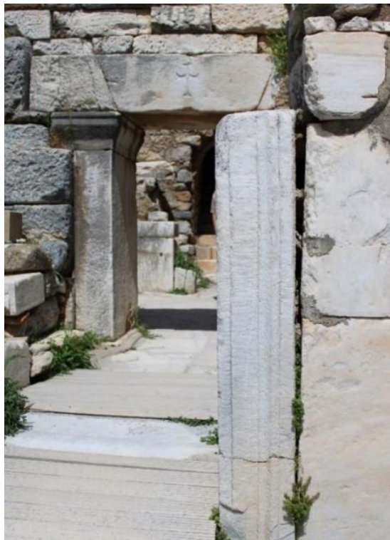
Figure 4.25. Cement infill between the entrance door block and cut stone (south) façade (Photograph: T. Tekin, 03.04.2022).
