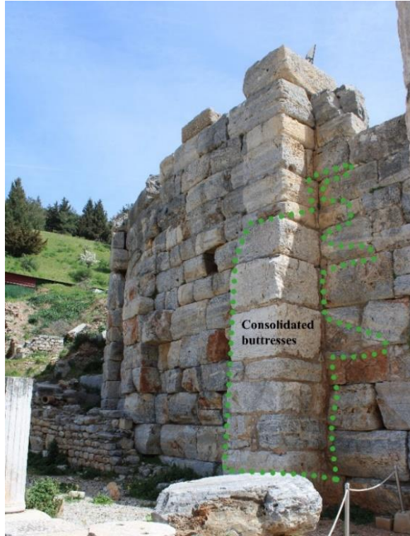
Figure 4.24. Consolidated buttress at the west side of the bouleuterion (Photograph: T. Tekin, 03.04.2022).
