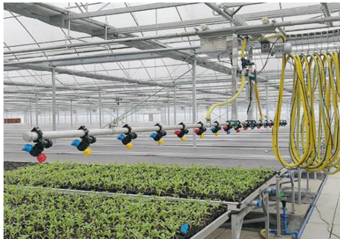
Figure 3.6. Irrigation System and Filter Systems for Sample Greenhouse Design (Courtesy of Emre İçöz)
