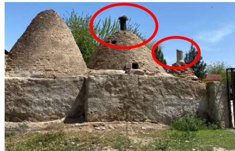
Figure 4.36. Illegal ventilation interventions, shown in red circles, to dome of houses (2021, April 16).
