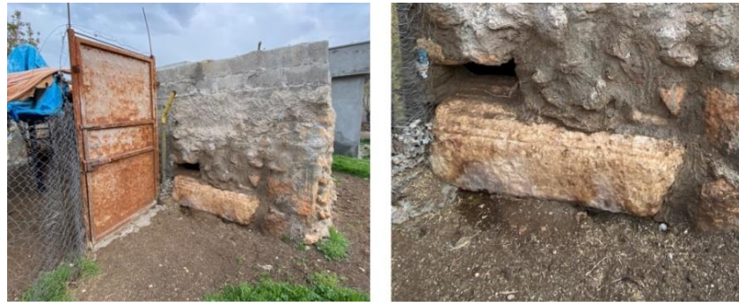
Figure 4.8. A piece of stone used on the wall of a traditional warehouse building, Ayanlar Tell (2021, April 12).
