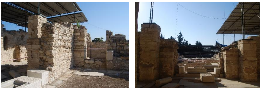
Figure 3.10. Bonding differences and discontinuity in joints between the naos walls and narthex buttresses
