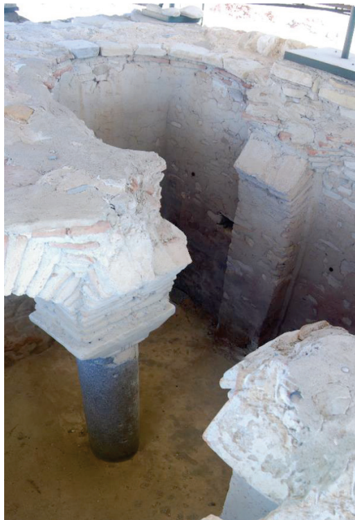
Figure 3.17. Photo of the cistern in the west corner showing the remains of arches and domes
