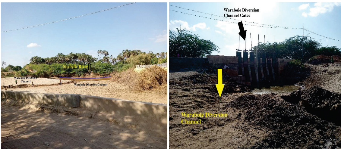
Figure 5.3 (c): Ongoing rehabilitation of the Warabole diversion channel at the downstream in the Right floodplain in the Study Area
