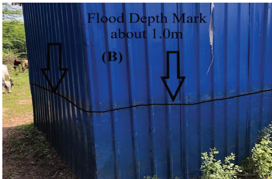
Figure 4.21 (b). The Observed flood depth mark of the Deyr 2019 flood at downstream in the city
