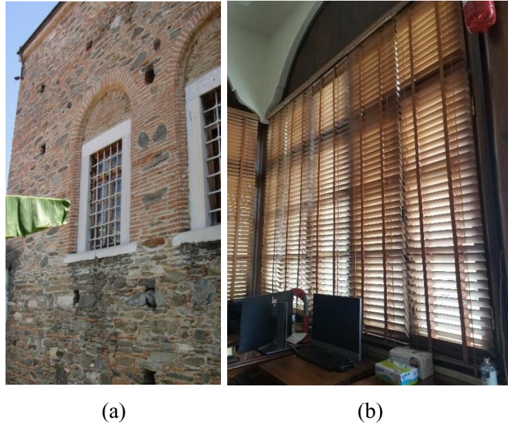
Figure 3.16. External walls of main hall (a) and office area (b) (Source: Umut Çağırğan archive, 2021)
