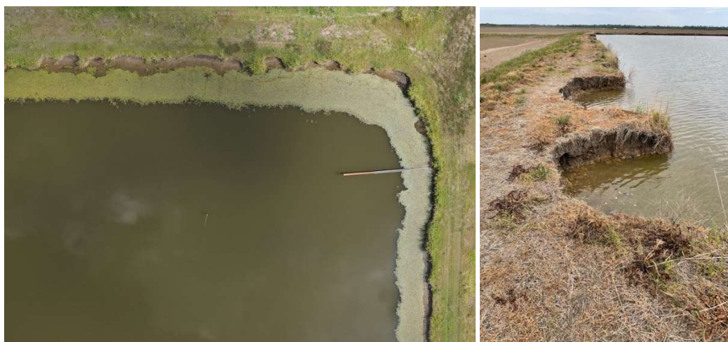
Figure 1. The northeast embankment of Johnson Farm reservoir near Shelby, MS
