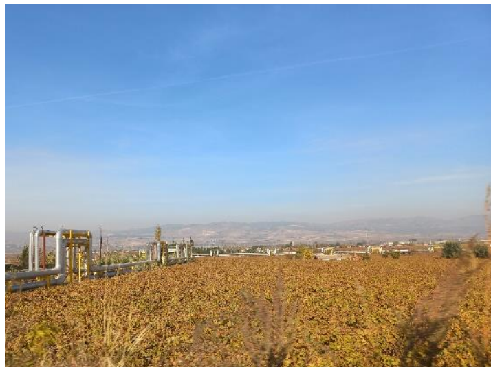
Figure 4.13. Pipelines of geothermal power plants in Piyadeler (Source: Taken by the author, 2021)
