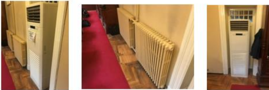
Figure 2. Air-conditioners and radiators used for the case building
