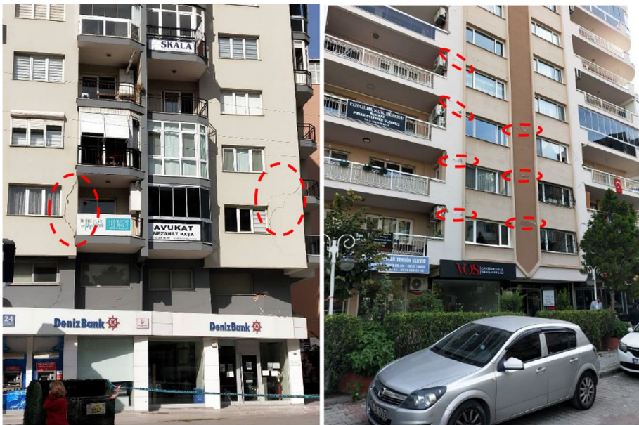
Fig. 16 Cracks in the non-structural walls due to the earthquake (wall cracks are shown with red dashed circles)
