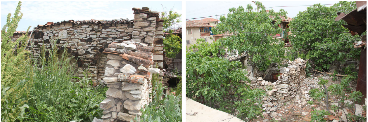
Figure 11. Ruined walls in two dwelling units located within the Rum neighbourhood.
