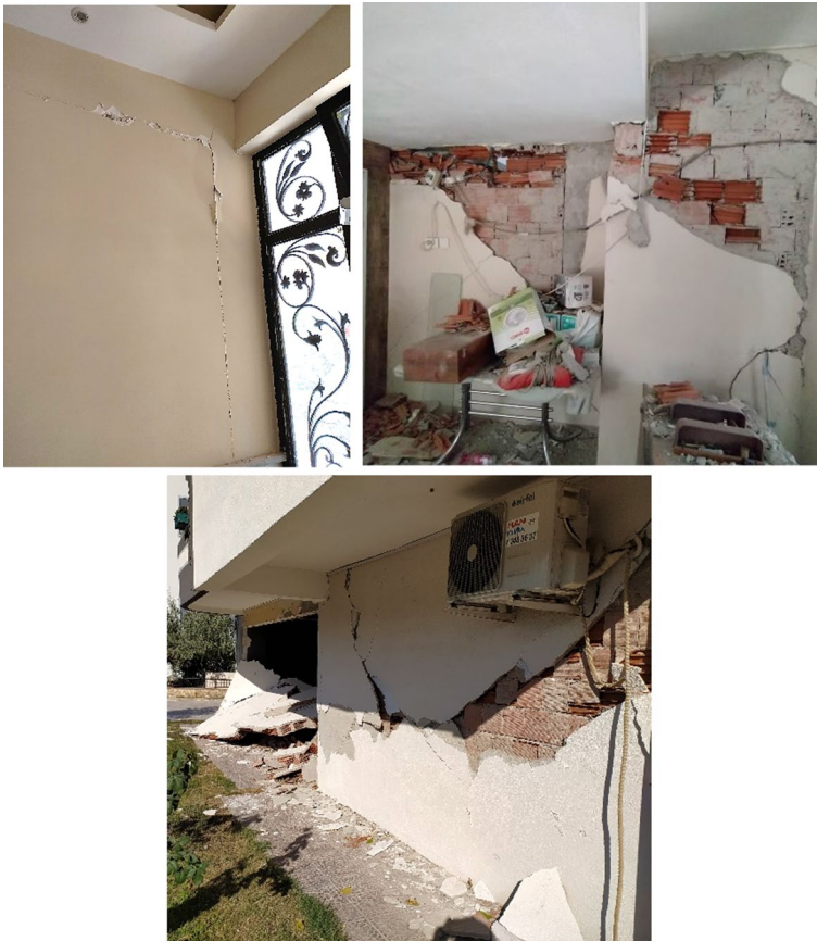
Fig. 8 Types of Infill wall damages observed in İzmir
