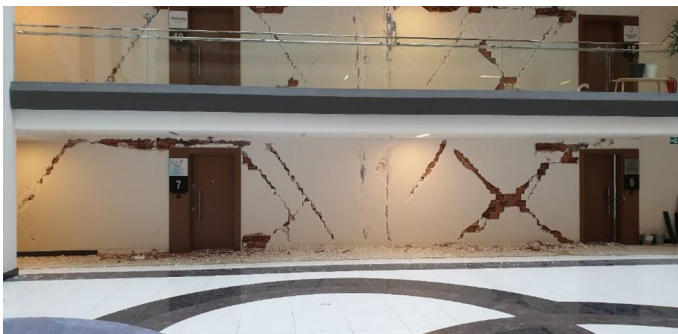
Fig. 13 Non-structural damage in infill walls due to large openings in the slab
