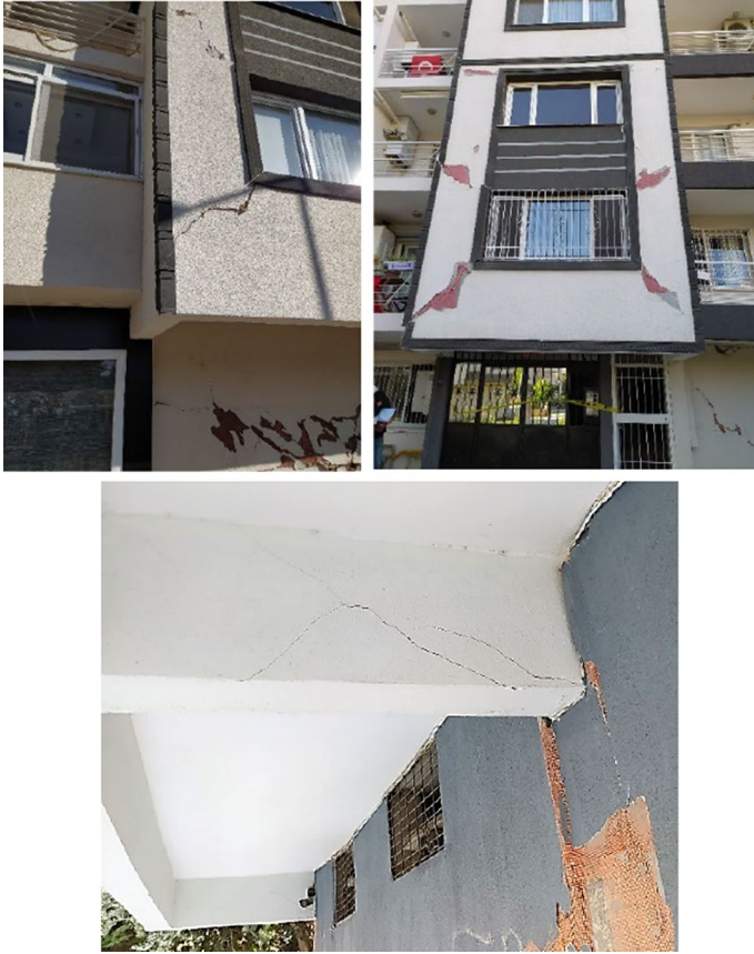
Fig. 10 Damage in overhangs
