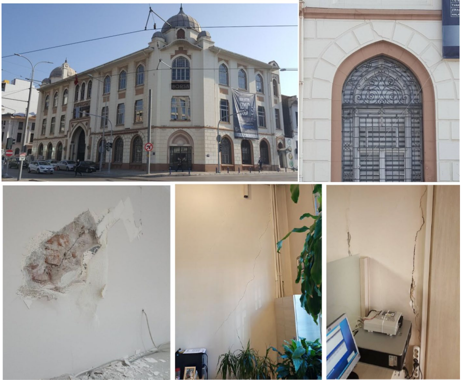
Fig. 14 İzmir commerce building: general view and observed damages
