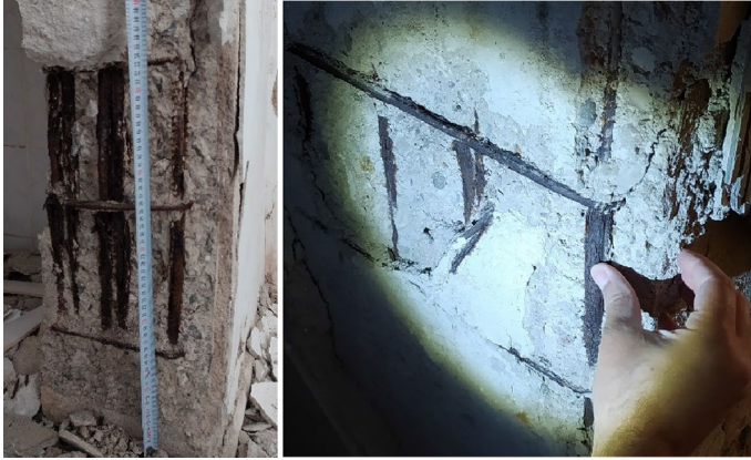
Fig. 12 Corrosion induced damages
