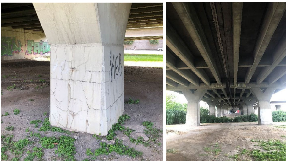
Fig. 21 ASR based cracks (non-seismic) and general view
