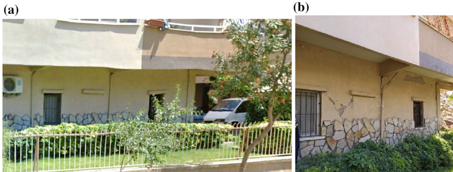
Fig. 9 Contribution of infill walls. a Before the earthquake (left), b after the earthquake (right)
