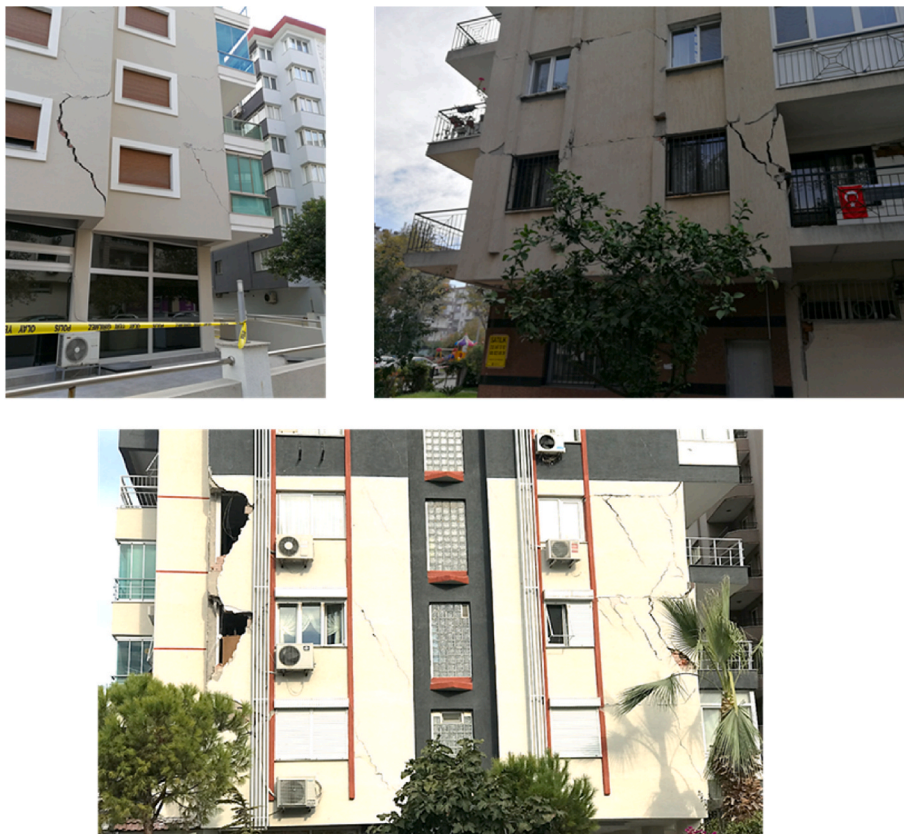
Fig. 23. Observed masonry wall damage due to the heavy overhangs.
