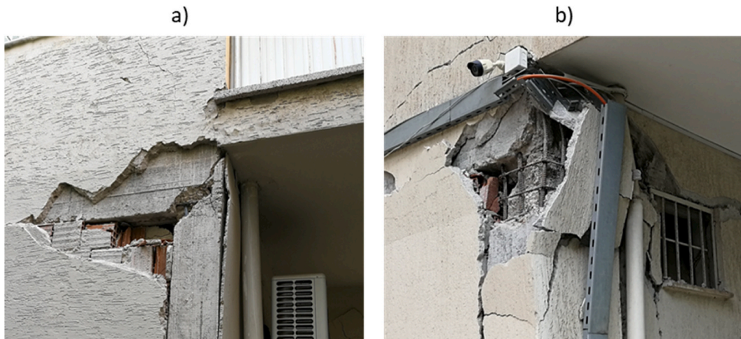
Fig. 20. a) Weak column-strong beam damage, b) Combined weak column-strong beam and shear failure.
