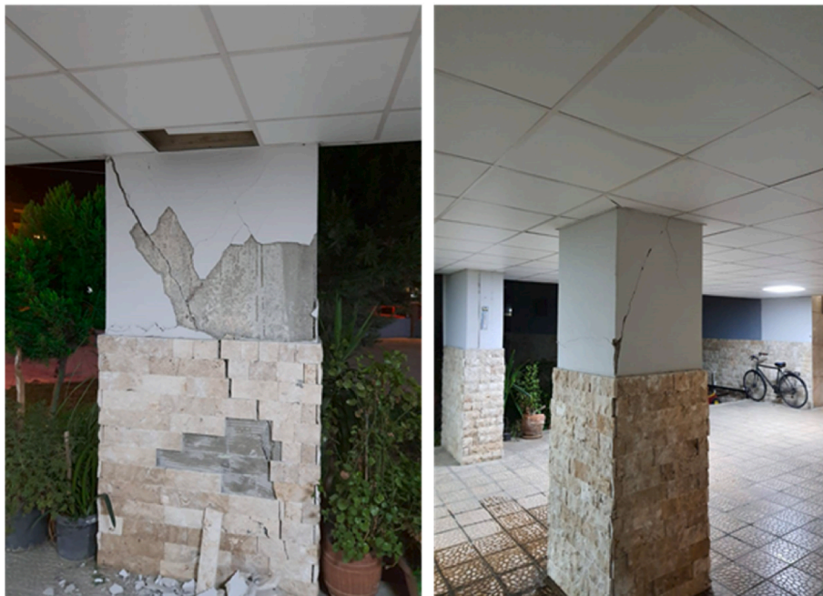
Fig. 21. Views from the observed soft story effect a) First story collapse [21]. b) shear damage.
