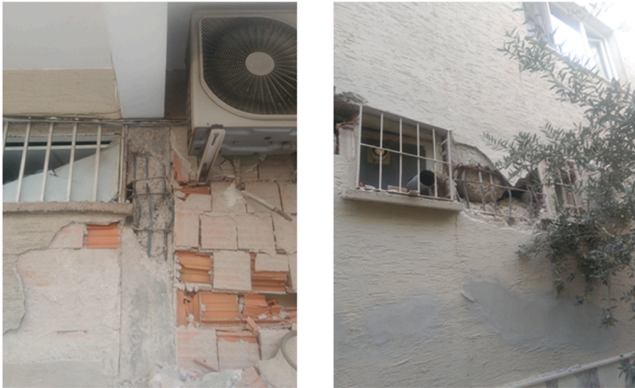
Fig. 22. Observed shear failures due to the short column effect.
