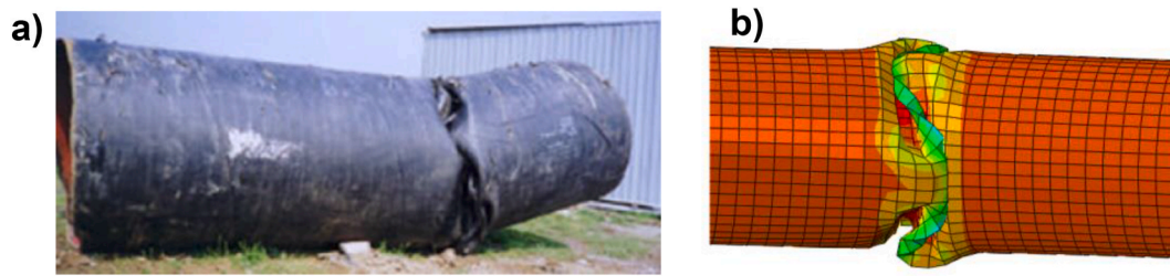
Fig. 22. a) Observed plastic deformations of the Thames water transmission pipe aftermath of the 1999 Kocaeli Earthquake (Kaya et al., 2017), b) calculated plastic deformations of the Thames water transmission pipeline.
