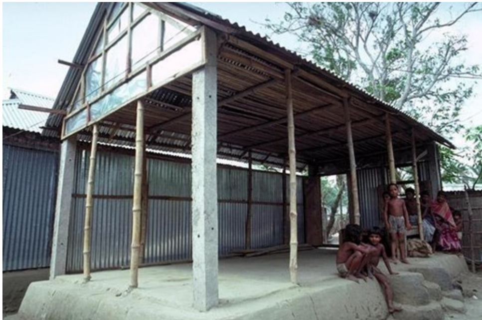
Figure 28. Image from the construction stage. Four concrete columns, a pre-fabricated sanitary slab and twenty six corrugated iron roofing sheets given under the loan. (Source: Archnet)
