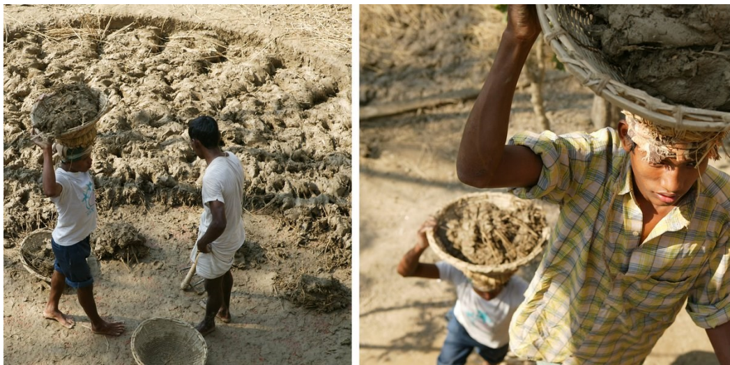
Figure 21. An image from the construction stage: The soil is mixed with straw.
