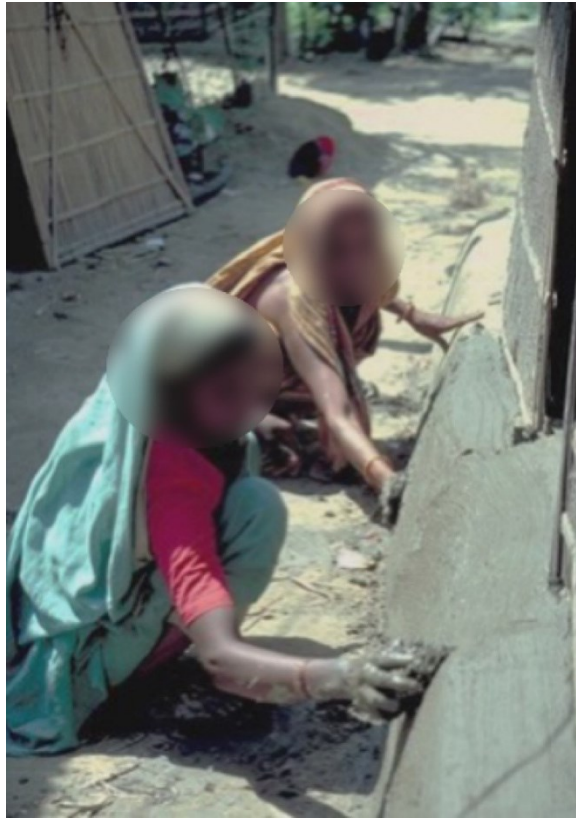
Figure 32. The construction of the cob ground together (Source: “Grameen Bank Housing Programme, Various locations, Banglades” Archnet)
