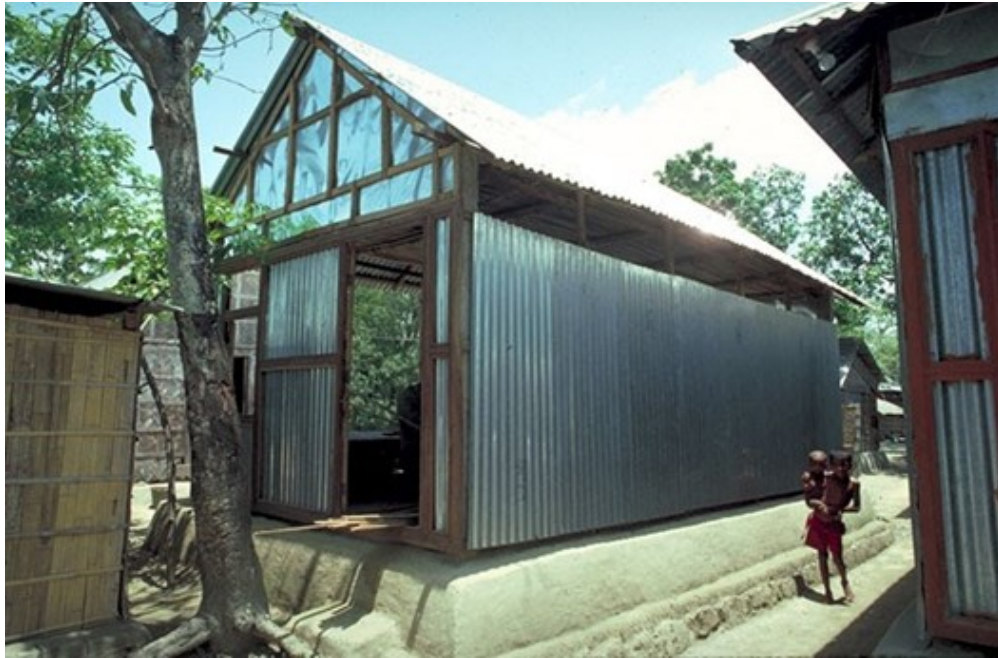
Figure 29. Image from the construction stage. Four concrete columns, a pre-fabricated sanitary slab and twenty six corrugated iron roofing sheets given under the loan. (Source: Archnet)
