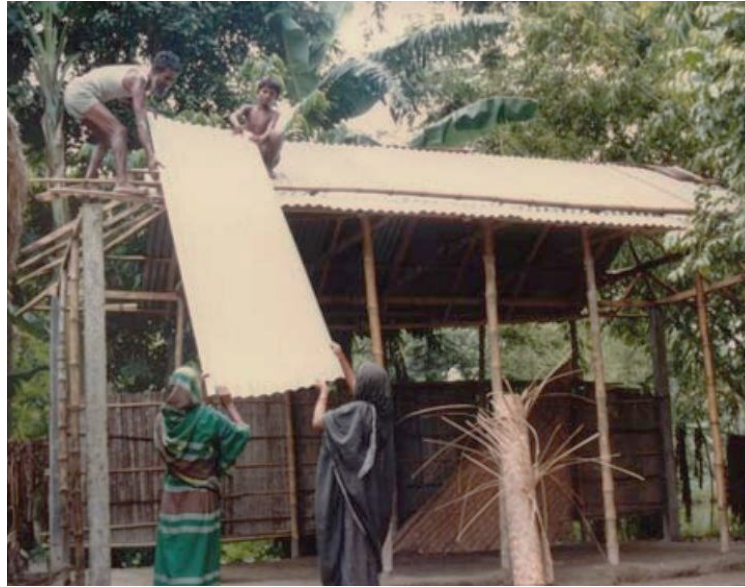
Figure 31. Neighbors placing the roof of the house together. (Source: “Grameen Bank Housing Programme, Various locations, Banglades” Archnet)
