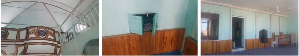
Figure 4. 15. Confessional booth and where the pipe organ used to be before the church was converted into a mosque.
