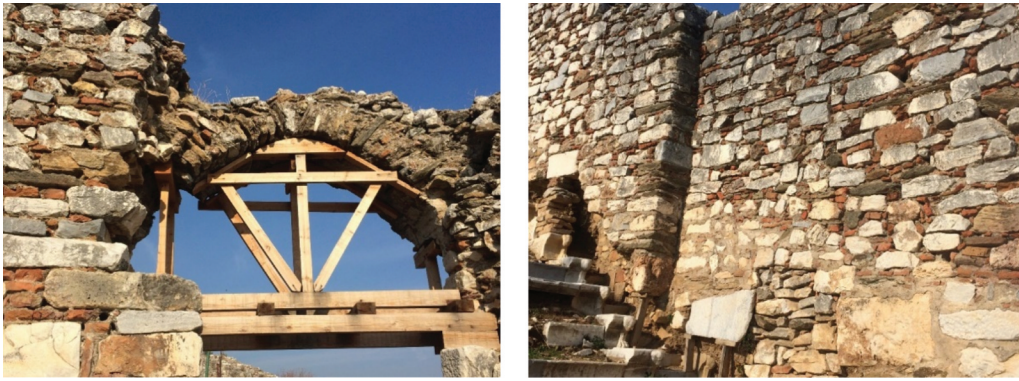
Figure 6. Consolidation of an arch (left), supporting of the walls (right) in the Bouleuterion, Metropolis, İzmir, Turkey.
