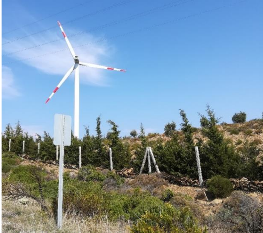
Figure 6. 8. Enclosed Wind Farm in Sarpıncık (Field Survey, October 2018)
