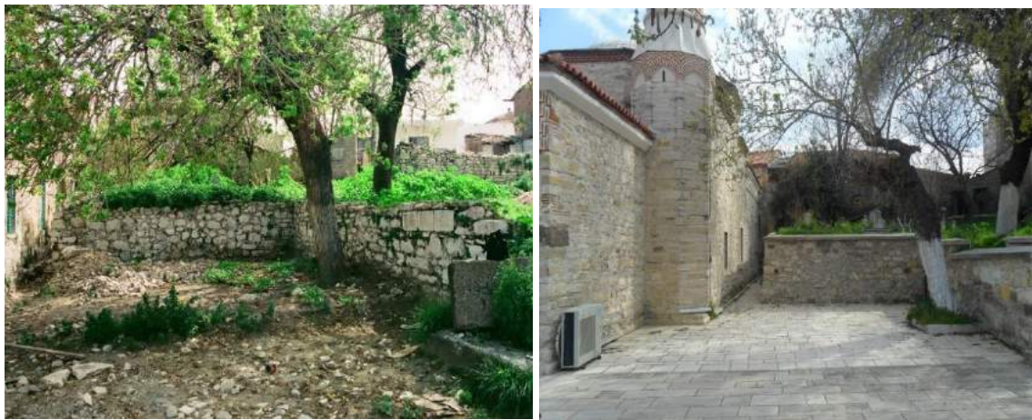
Figure 3.70. The Kapan Mosque courtyard before (left) (Source: RDPF Archive, 1990) and after restoration implementation as viewed from the southwest
