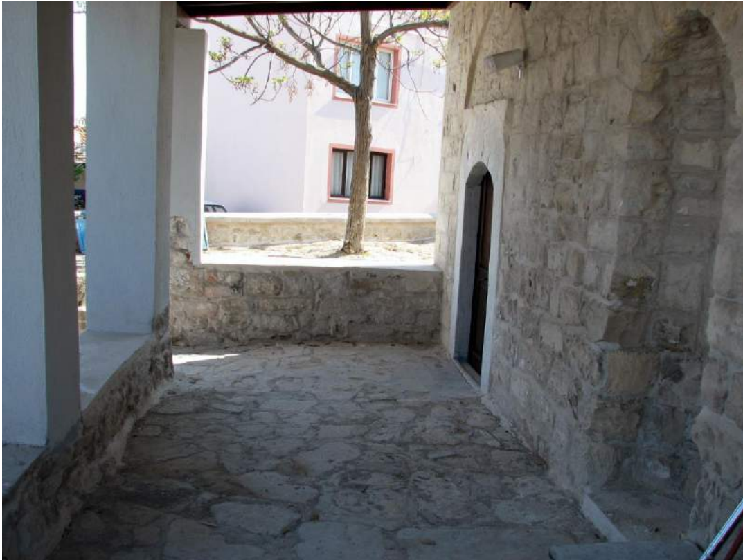
Figure 3.52. The Last comers' hall interior as viewed from southwest after restoration (Source: RDPF Archive, 2006)
