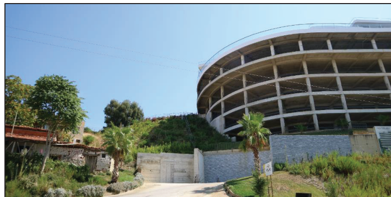
Figure 5.23. Vitalia project during the construction stage rising next to the squatter housing
