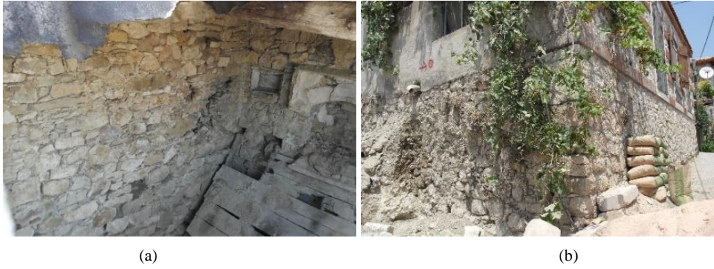
Figure 4.1. Stone masonry foundation (a) in Eğlenhoca (By author, October 2016), (b) İncecik (June 2016).
