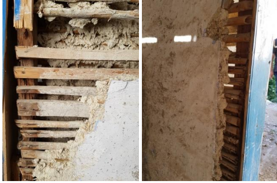
Figure 4.27. Timber Framed Wall Example in İncik (June 2017).
