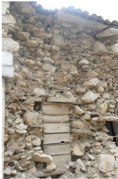
Figure 4.102. Example of Cupboard Placed in a Niche; View of Back Side (June 2016).
