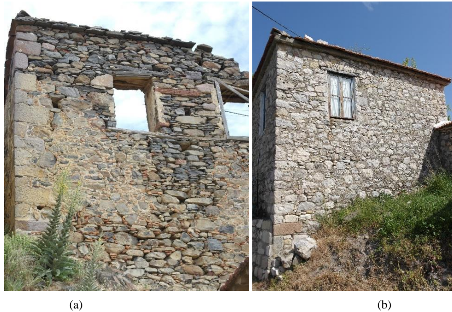
Figure 4.3. Stone masonry wall (a) in Küçükbahçe (By author, April 2017), (b) in Kösedere (April 2017).
