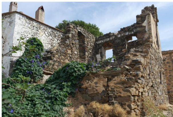
Figure 1.3. Disappearing structures in Salman (October 2016).
