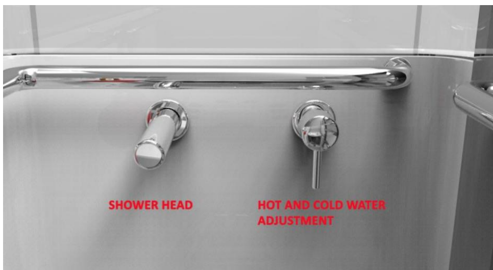
Figure 4.42. Showerhead and hot-cold water adjustment handle.
