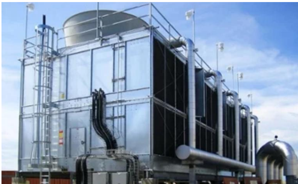
Figure 4.11. Commercial Cooling Tower [65]
