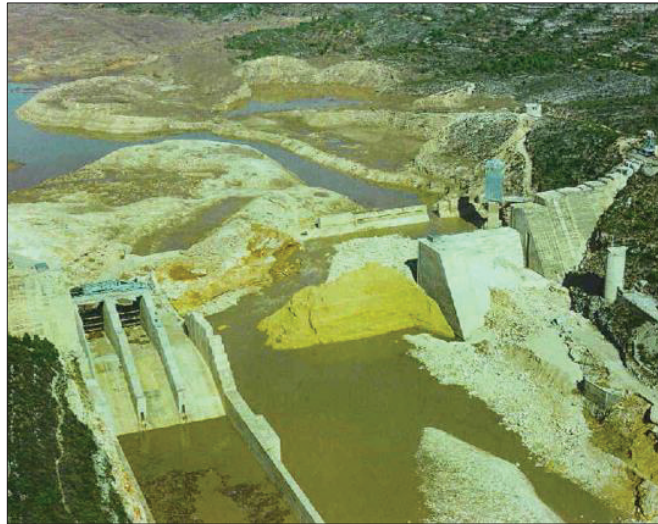
Figure 1.2: Tous Dam Failure (Source: Alcrudo, 2003)
