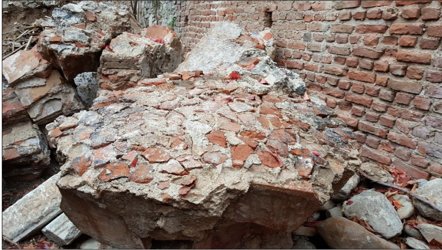
Figure A.59. The dome ruins and horasan plaster layer with crushed bricks (Source: Fatma Gürhan, December 2016)
