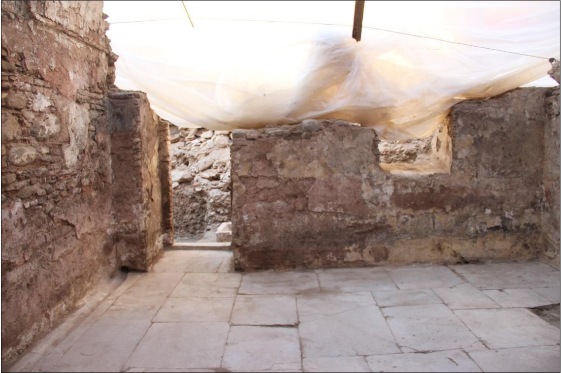
Figure A.77. The opening and a niche on the northwest wall (Source: Mükerrerem Kürüm archive, May 2017)
