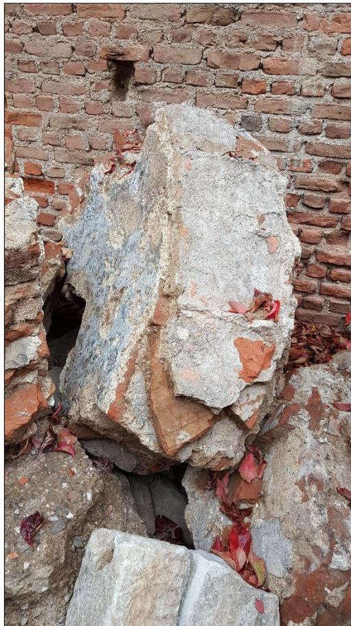
Figure A.60. The dome ruins and horasan plaster layer with crushed bricks (Source: Fatma Gürhan, December 2016)
