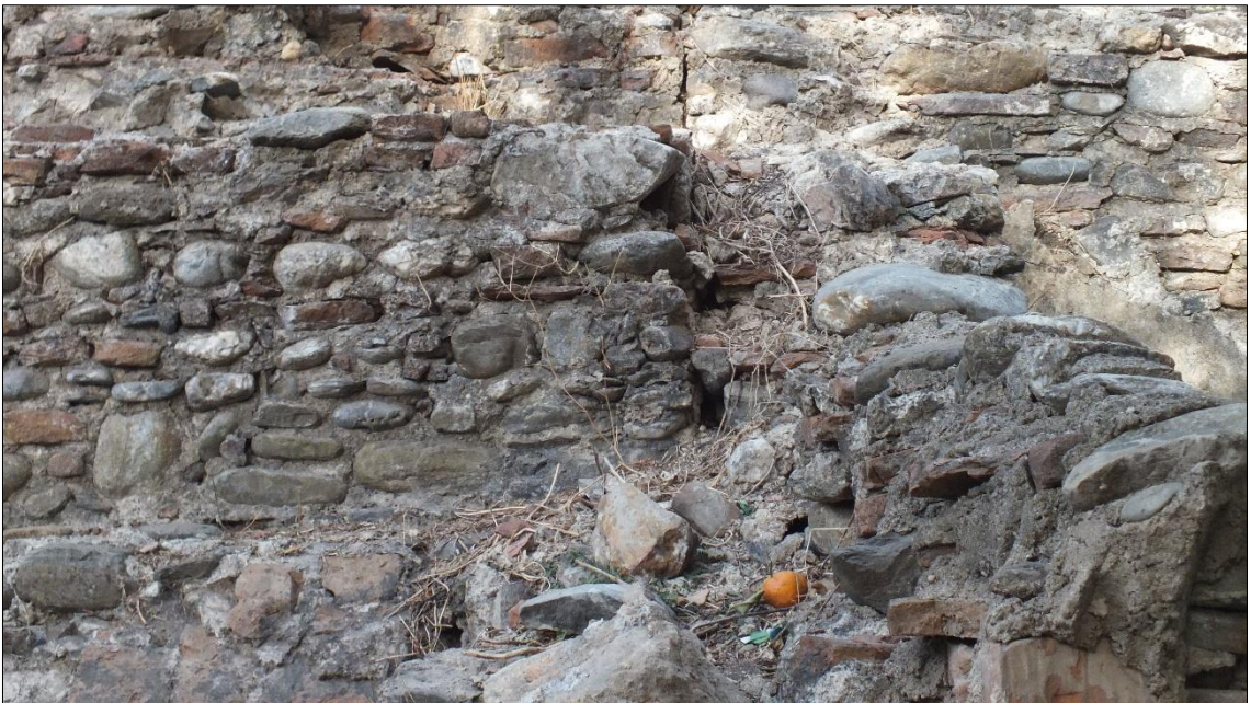
Figure A.82. The junction line between the hot water reservoir and soyunmalık-ılıkık wall (Source: ANKA Architecture and Restoration Office archive, October 2016)
