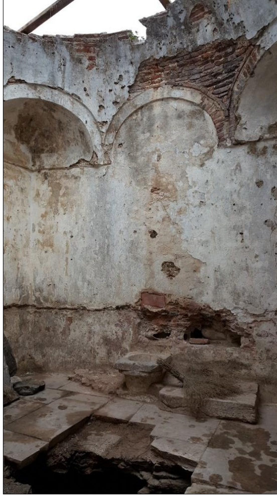
Figure 2.11. Eski Hamam G02 Sıcaklık (Source: Fatma Gürhan, December 2016)
