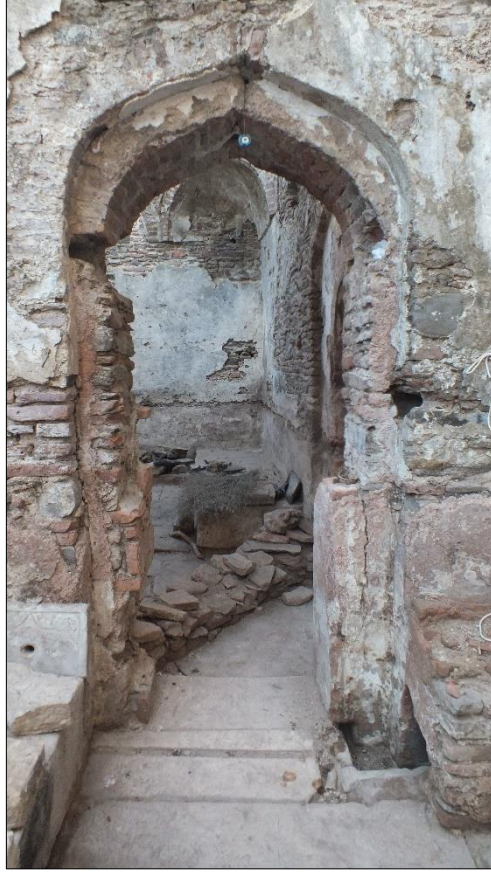
Figure A.41. Transition from the soyunmalık-ılıklik to the sıcaklık space (Source: ANKA Architecture and Restoration Office archive, November 2016)
