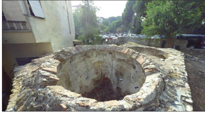
Figure A.56. The dome remain of G02 Sıcaklık (Source: ANKA Architecture and Restoration Office archive, July 2016)
