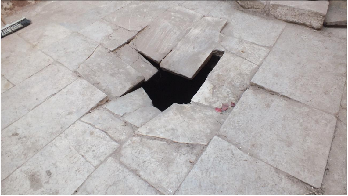
Figure A.54. The floor covering of the G02 Sıcaklık space (Source: ANKA Architecture and Restoration Office archive, November 2016)
