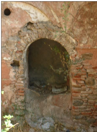
Figure A.76. The brick set at the transition between G03 Sıcaklık and G04 Sıcaklık (Source: Mükerrerem Kürüm archive, May 2017)
