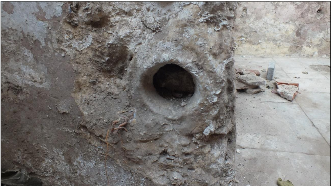
Figure A.78. The interrupted terracotta pipe in the opening on the northwest wall (Source: Mükerrerem Kürüm archive, May 2017)
