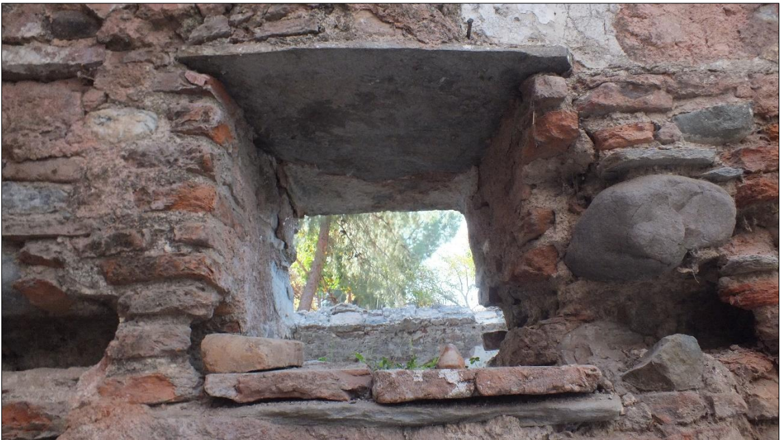
Figure A.74. The control window at the wall of G04 Sıcaklık (Source: ANKA Architecture and Restoration Office archive, November 2016)
