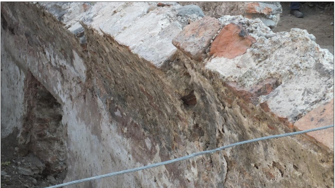
Figure A.80. The junction line between the vaults with different pitches (Source: ANKA Architecture and Restoration Office archive, November 2016)
