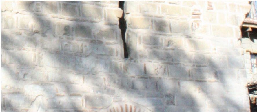
Figure 3.33. A detail from the southern façade showing a row of brick alternating with a cut stone row with a vertical brick between the stones in masonry technique.
