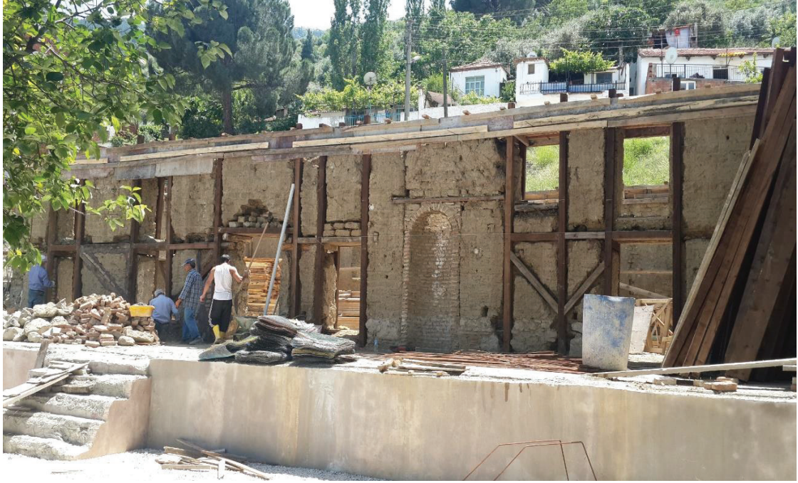
Figure 3.7. Northern wall of the prayer hall as viewed in the restoration of 2014, Haki Baba Mosque. (Source: Erturan 2012)
