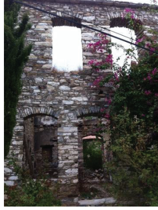
Figure 2.3. Restoration of a traditional building in abandoned old Doğanbey village in Söke, Aydın following the declaration as landslide zone. (Source: Büyükkılıç-Koşun 2014)
