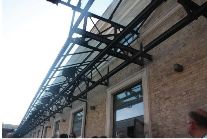
Figure 2.10. Eave addition to historic mansion converted into auditorium, Faculty of Architecture, Roma Tre University, Rome. (Source: Hamamcioğlu-Turan 2018)
