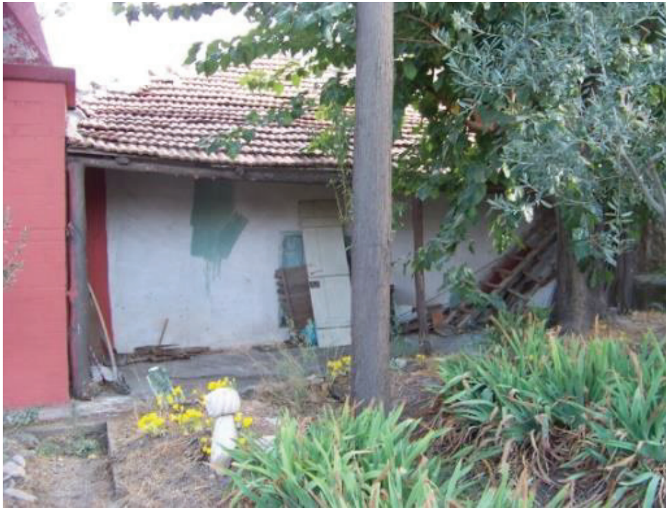
Figure 3.8. Post remains carrying the eave at the Haki Baba Mosque (Source: RDPF 2012)
