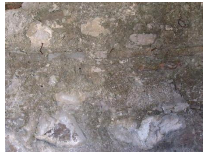
Figure 4.38. Pittings and microbiological colonizations on the right part
