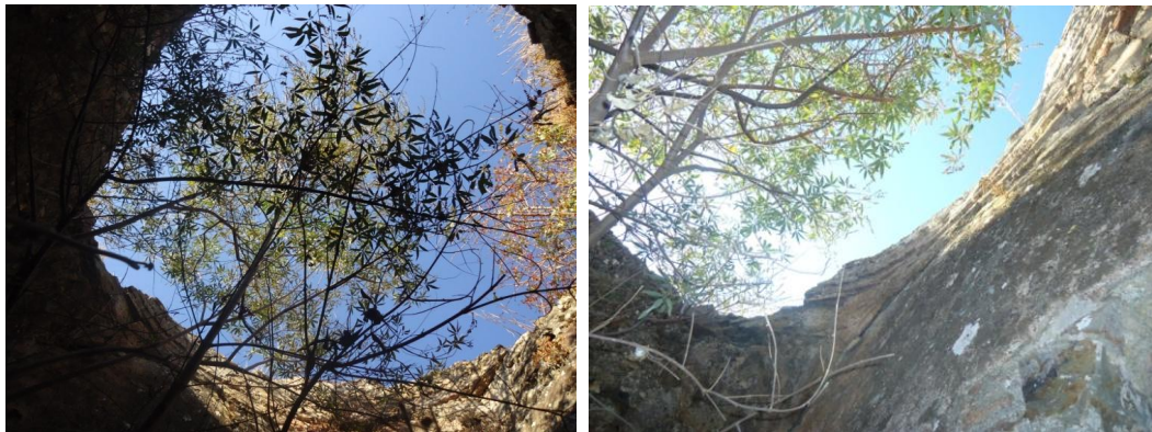
Figure 4.178. Dome plaster of the South West Halvet
