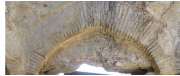
Figure 4.40. Deformation on the West arch
