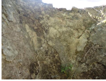
Figure 4.177. South West pendentive plaster of the South West Halvet
