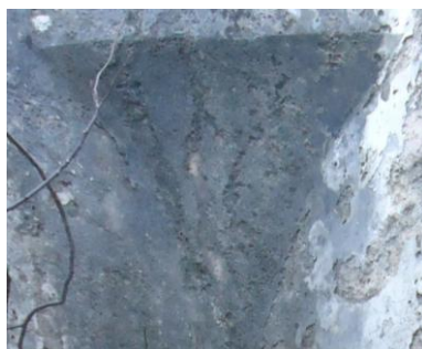
Figure 4.129. South West pendentive of Cleaning Cell
