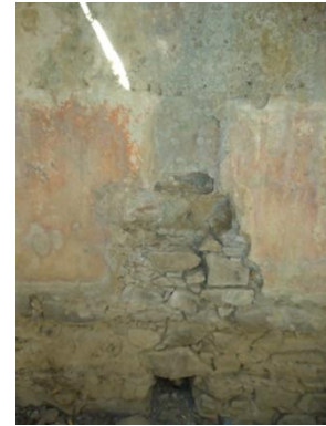
Figure 4.88. Missing part of the wall
