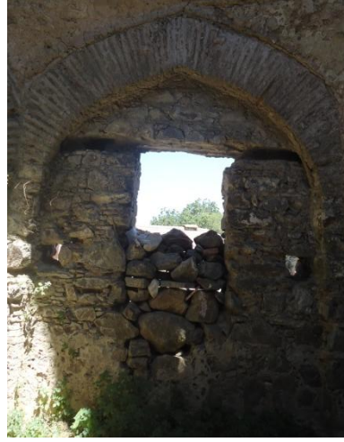
Figure 4.68. North arch plaster of Soyunmalık
