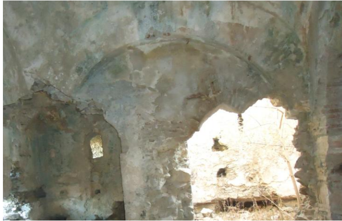
Figure 4.112. South Arch plaster of Sıcaklık
