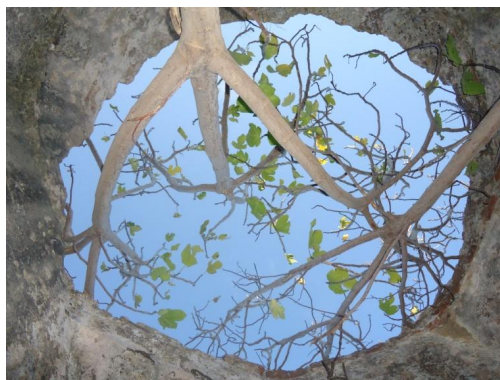
Figure 4.131. Dome of Cleaning Cell
