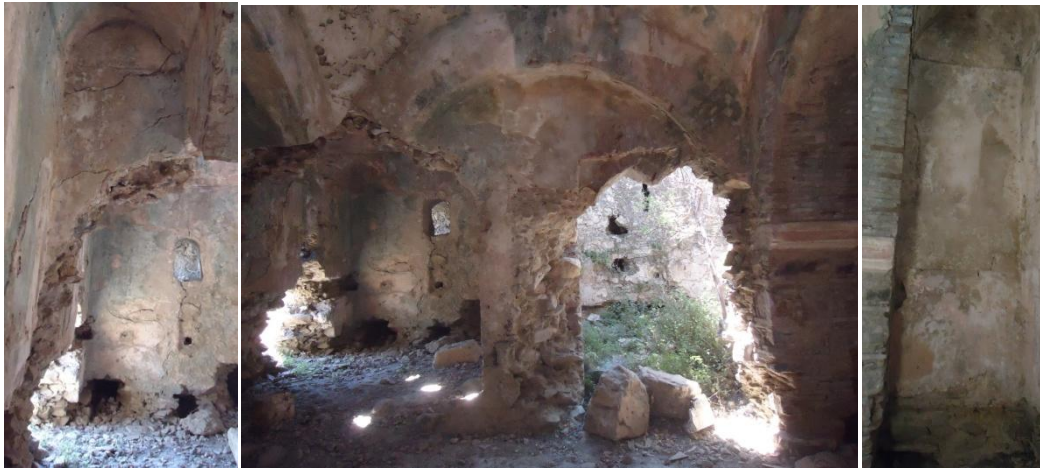
Figure 4.108. South Wall plaster of Sıcaklık
