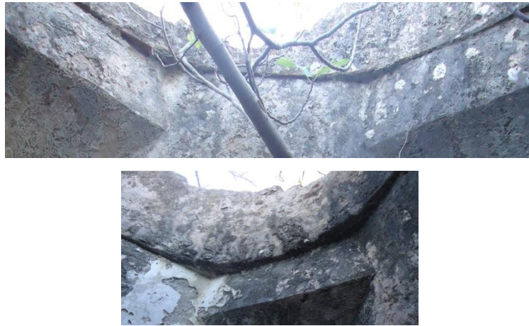
Figure 4.130. Drum of Cleaning Cell
