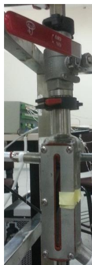
Figure 5.15. The relief valve between the adsorbent bed and evaporator tank after the revision of experimental setup.
