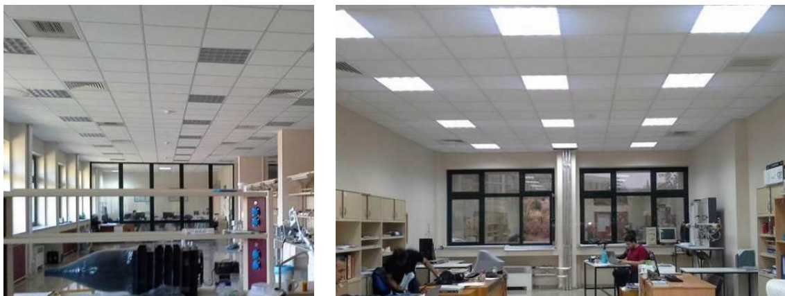
Figure 3.15 Luminaires in the building
