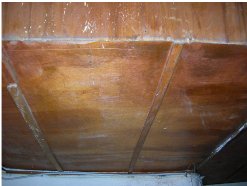
Figure 5.2. The plywood ceiling covering of the space under the stairwell which should be removed.
