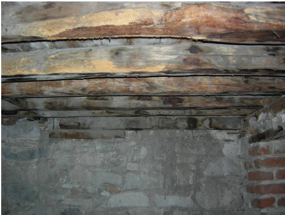
Figure 5.7. The deteriorated timber beams that are suggested to be replaced with chemically protected timber beams.
