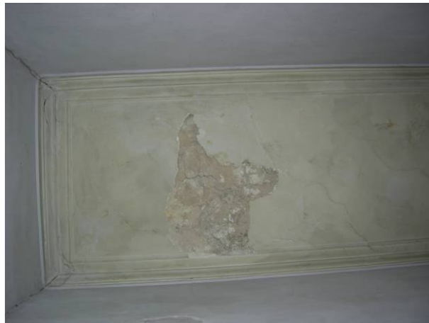
Figure 5.9. The plaster that is suggested to be replaced with plaster in original composition.
