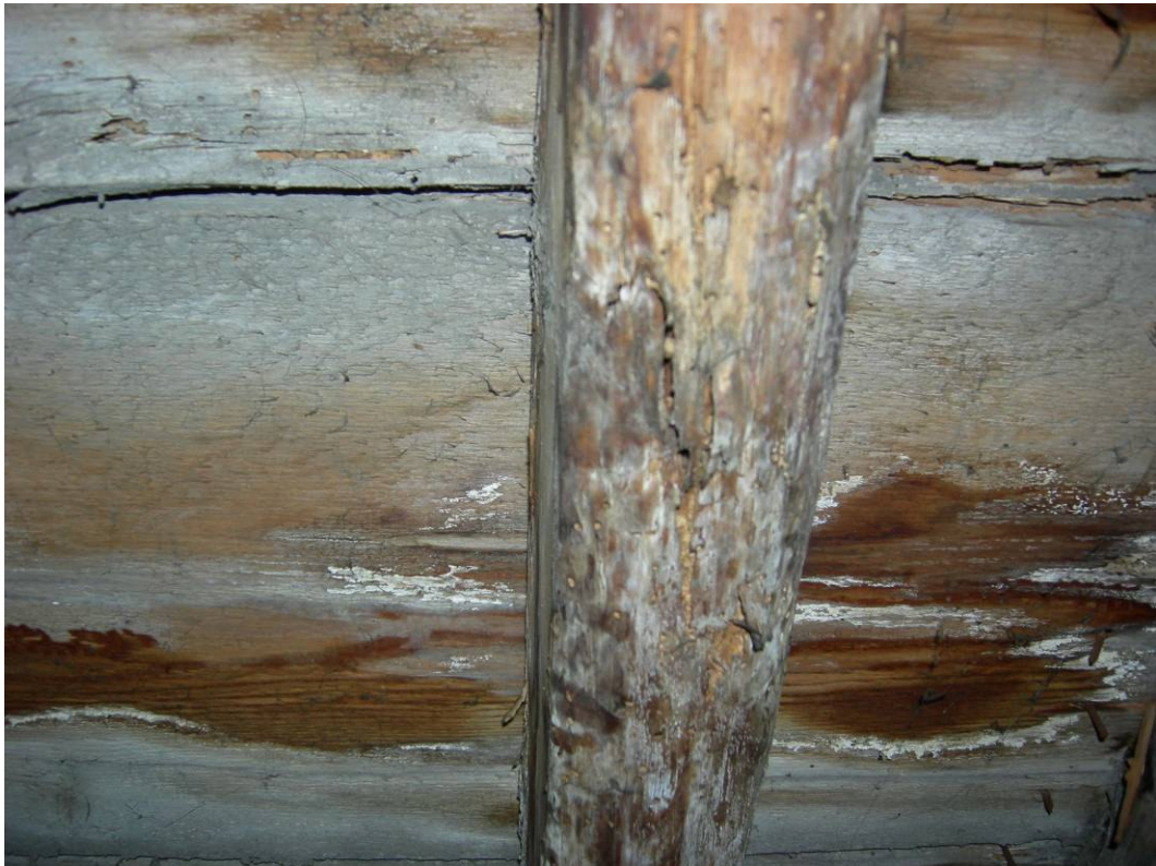
Figure 2.125. Holes in the timber beam, white stains in the timber covering at the basement.
