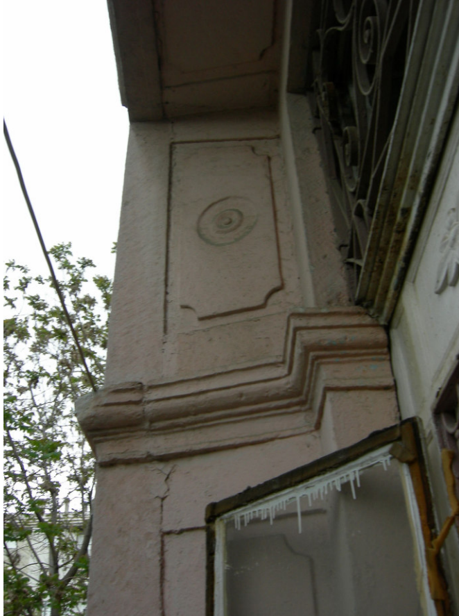
Figure 2.80. Decorative motifs on the lateral walls of the semi open entrance space.
