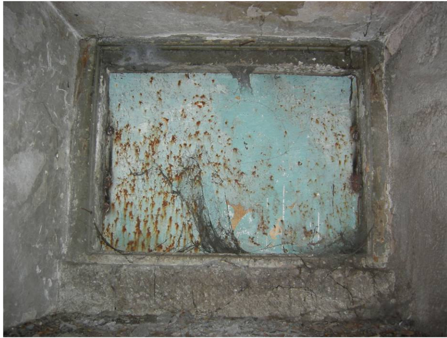
Figure 2.130. The heavily damaged iron shutters at the basement.
