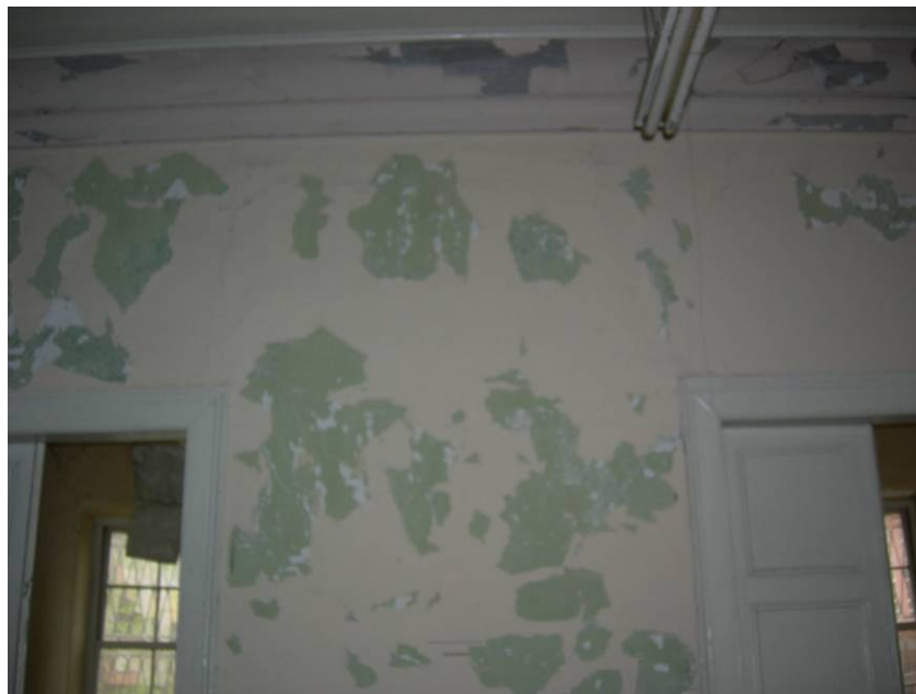
Figure 2.131. The loss of top layer paint on the walls of the hall at the ground floor.
