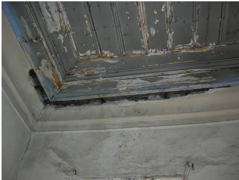
Figure 2.137. The deteriorated gypsum molding and the timber coverings of the ceiling of room 6.
