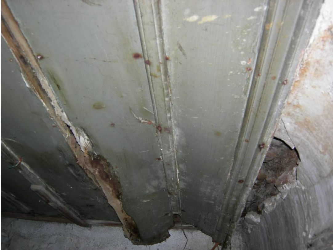
Figure 2.126. The deteriorated gypsum moldings and timber coverings at the basement.
