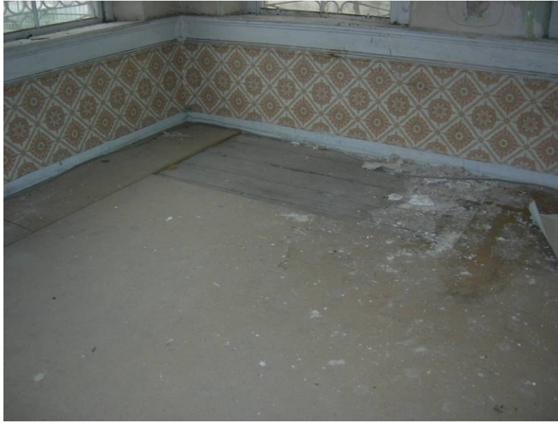
Figure 5.1. The additional chipboard coverings on the floor of room 1, 2 and 3 which should be removed.
