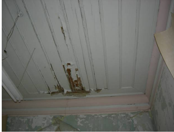
Figure 5.8. The deteriorated wood laths that are suggested to be removed.
