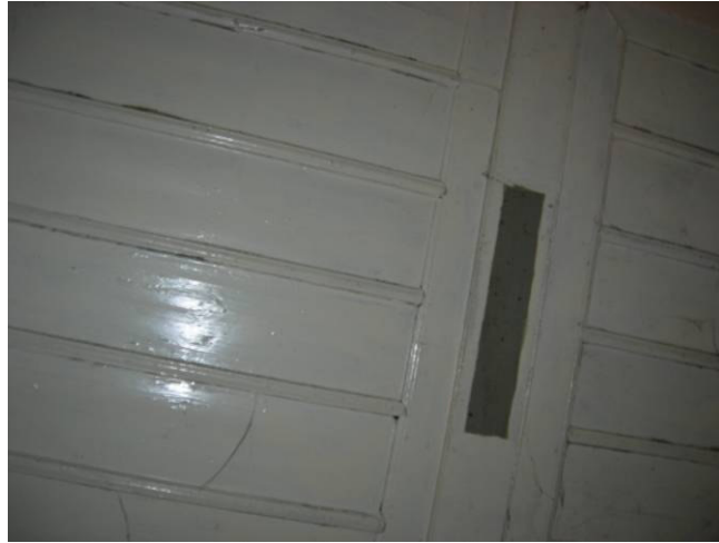
Figure 4.14. The trace of a separator on the ceiling of wet space at the first floor.
