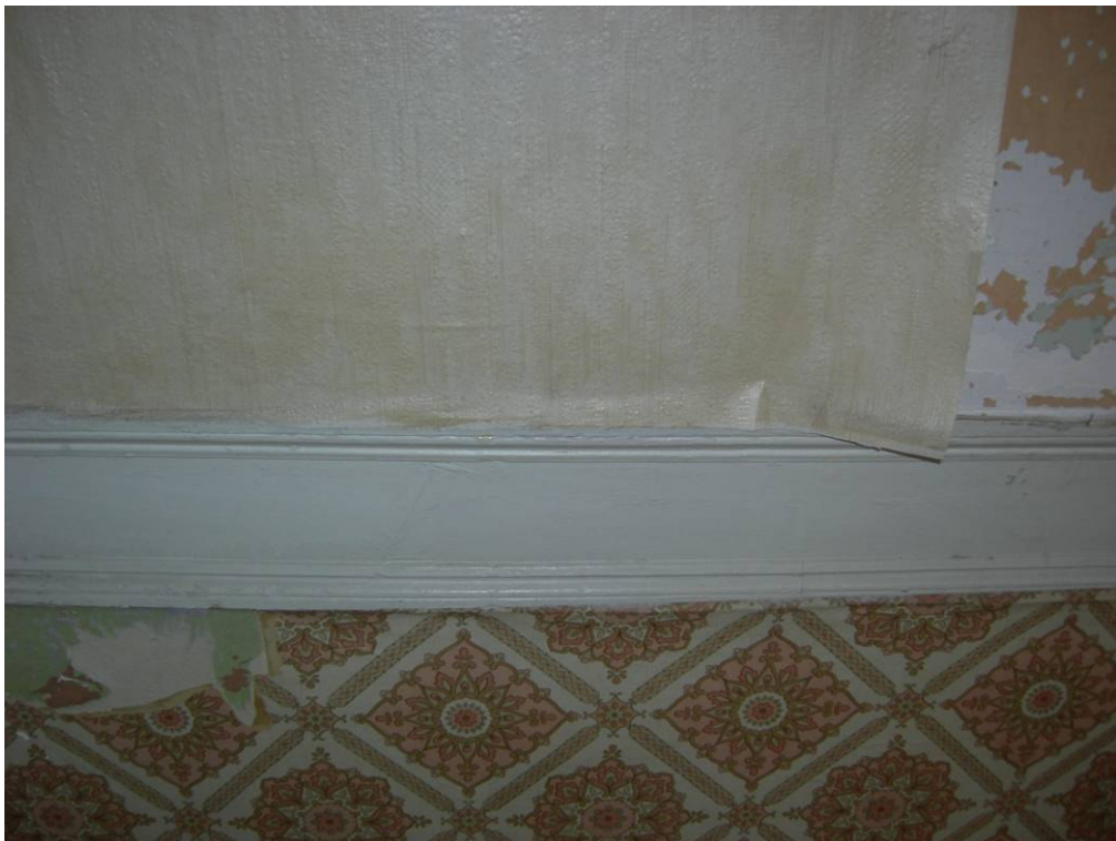
Figure 2.36. The timber chair rail running along the walls of room 2 at the ground floor.
