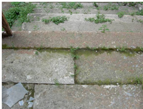
Figure 5.13. The rust stains on the stone that are suggested to be cleaned.
