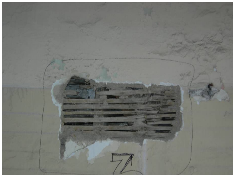
Figure 2.109. The interior timber skeleton walls covered with wood lath and mud plastered at the first floor.
