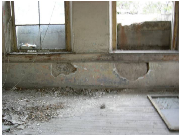
Figure 5.12. The deteriorated plaster on the east wall of room 6 that must be replaced
