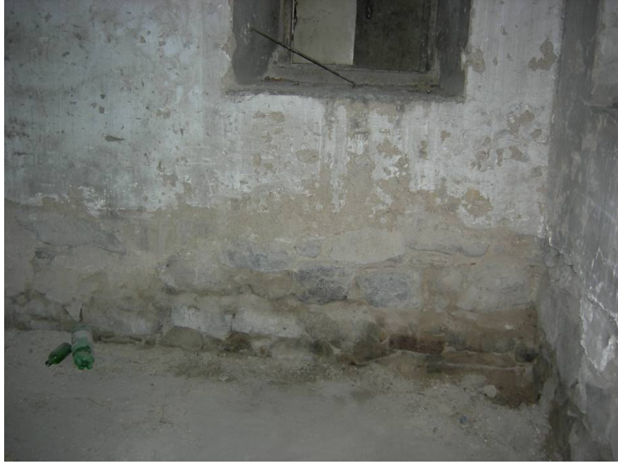
Figure 2.122. Loss of plaster on the interior walls of the basement.
