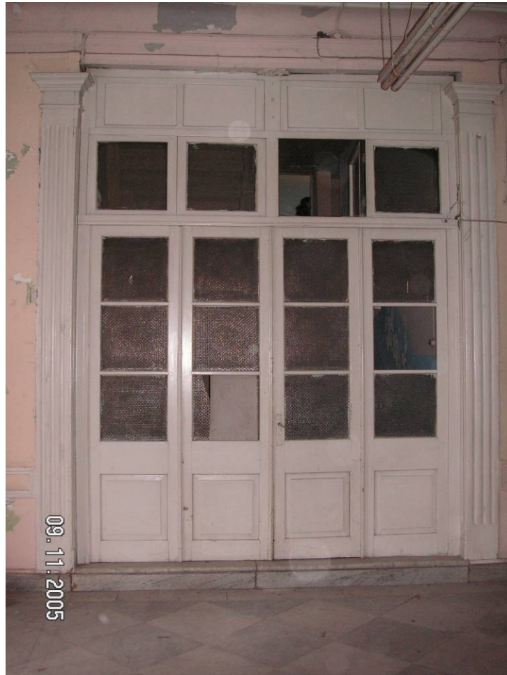
Figure 2.29. The arrangement of the opening between the inner hall and the stairwell.
