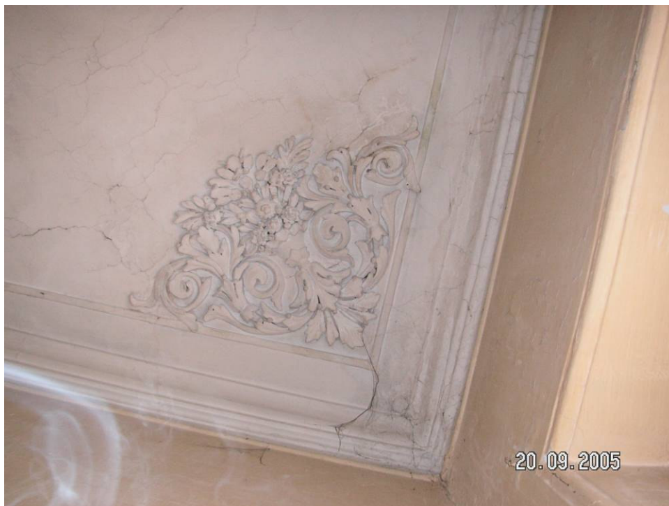
Figure 2.61. The molding and the stucco work at the corner of the ceiling of the hall at the first floor.
