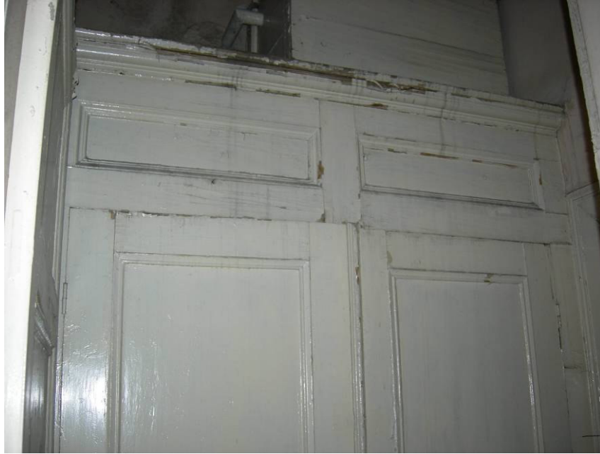
Figure 2.72. The cupboard in the connection space at the first floor.
