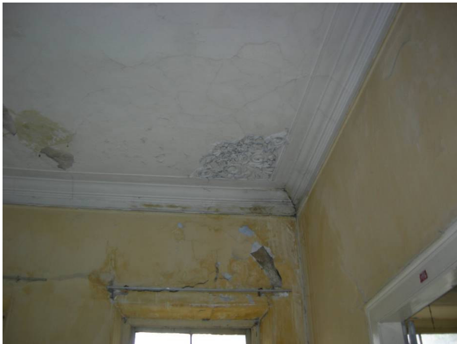
Figure 2.133. The deteriorated walls and ceiling of the hall at the first floor.
