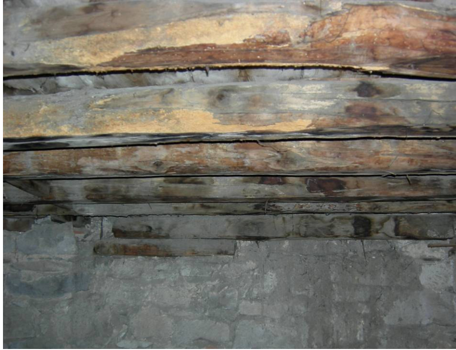
Figure 2.124. The deteriorated timber beams.
