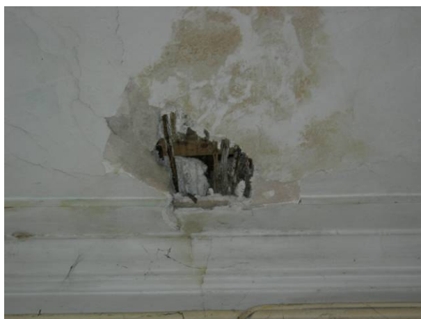
Figure 5.10. The plaster and the deteriorated wood laths that are suggested to be removed.
