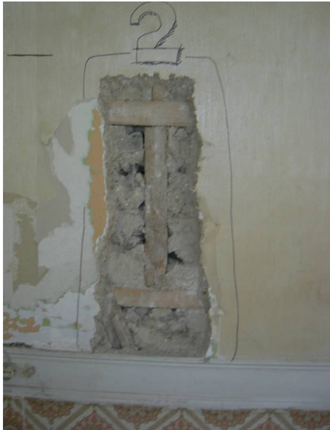
Figure 2.108. The stone infill of the timber skeleton interior walls at the ground floor of the house.
