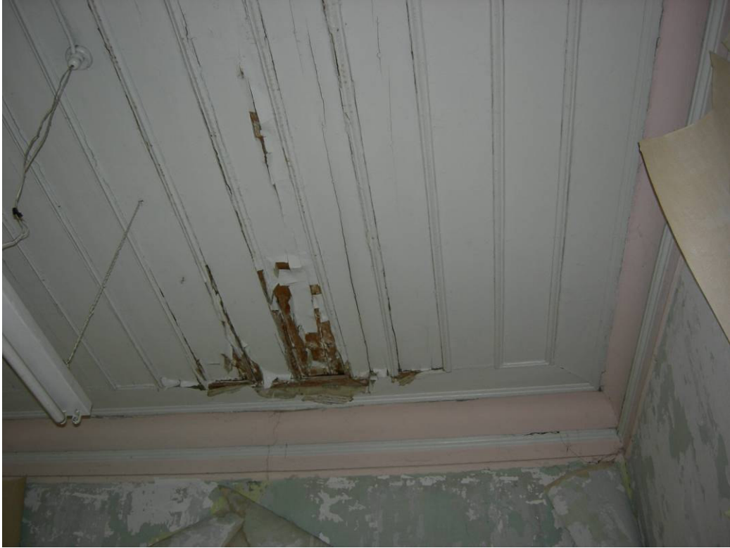
Figure 2.132. Loss of paint and timber decay on the ceiling coverings of room 1 at the ground floor.
