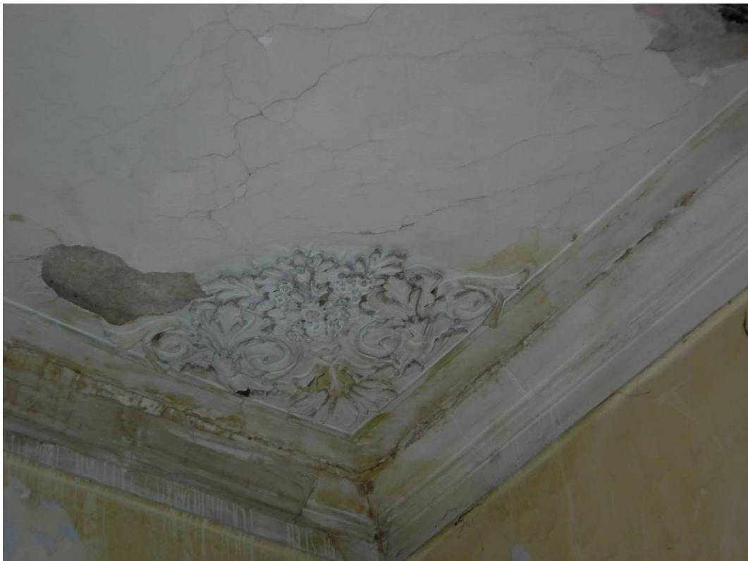
Figure 2.135. The partially detached ornaments on the ceiling of the hall at the first floor.
