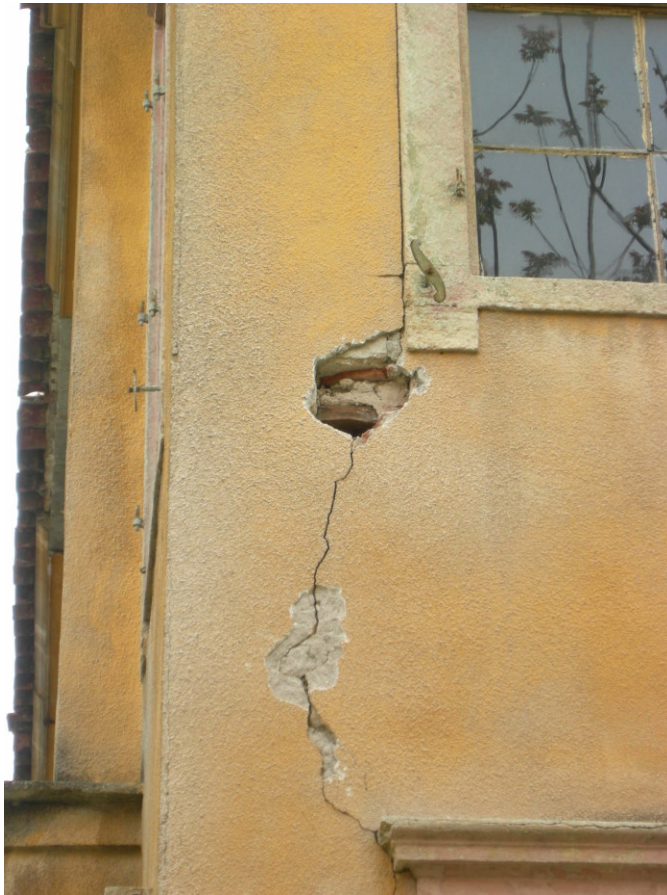
Figure 2.118. The major crack at the bottom level of the window at the northern corner of the western facade.
