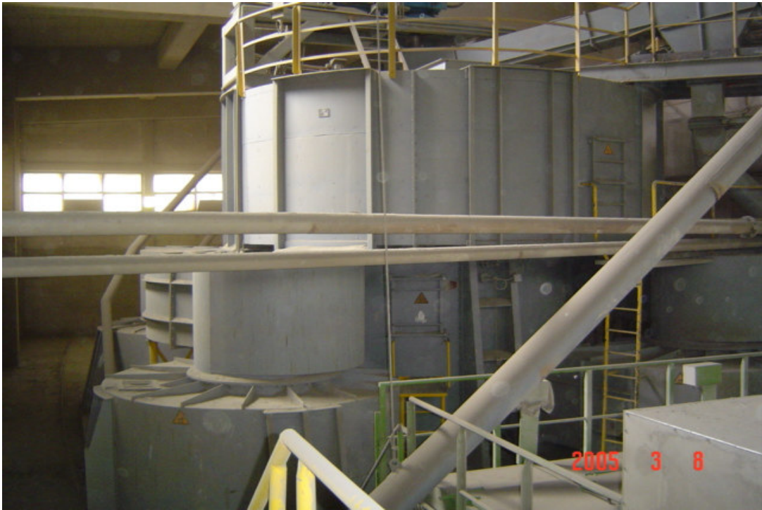
Figure B.4. Polysius® Cyclone Air Separator used in the local plant.
