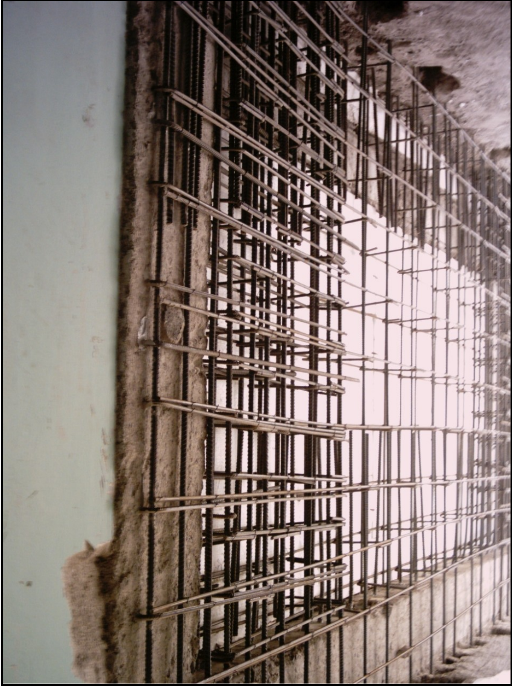
Figure 6.6. A New Shear Wall (Courtesy of Rehber Yapı Denetim San. ve Tic. A.Ş.)
