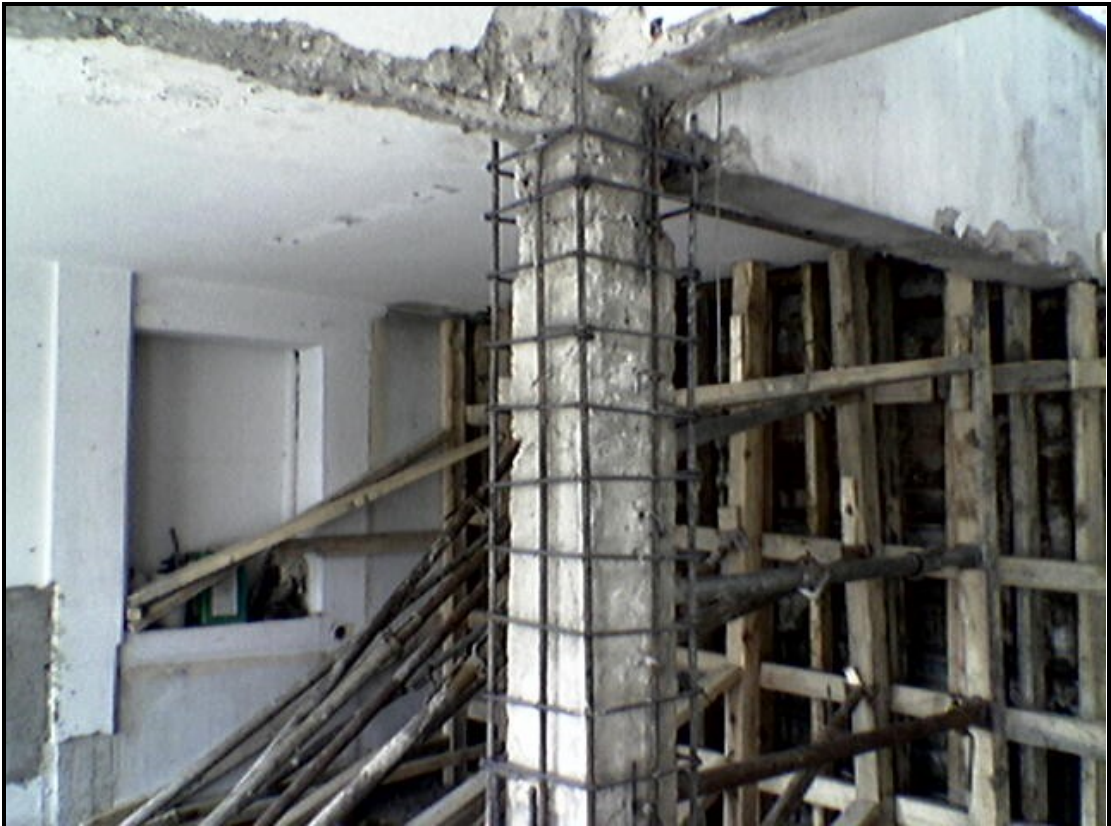
Figure 6.3. A Rehabilitated Column by using Jacketing Method (Courtesy of Rehber Yapı Denetim San. Ve Tic. A.Ş.)
