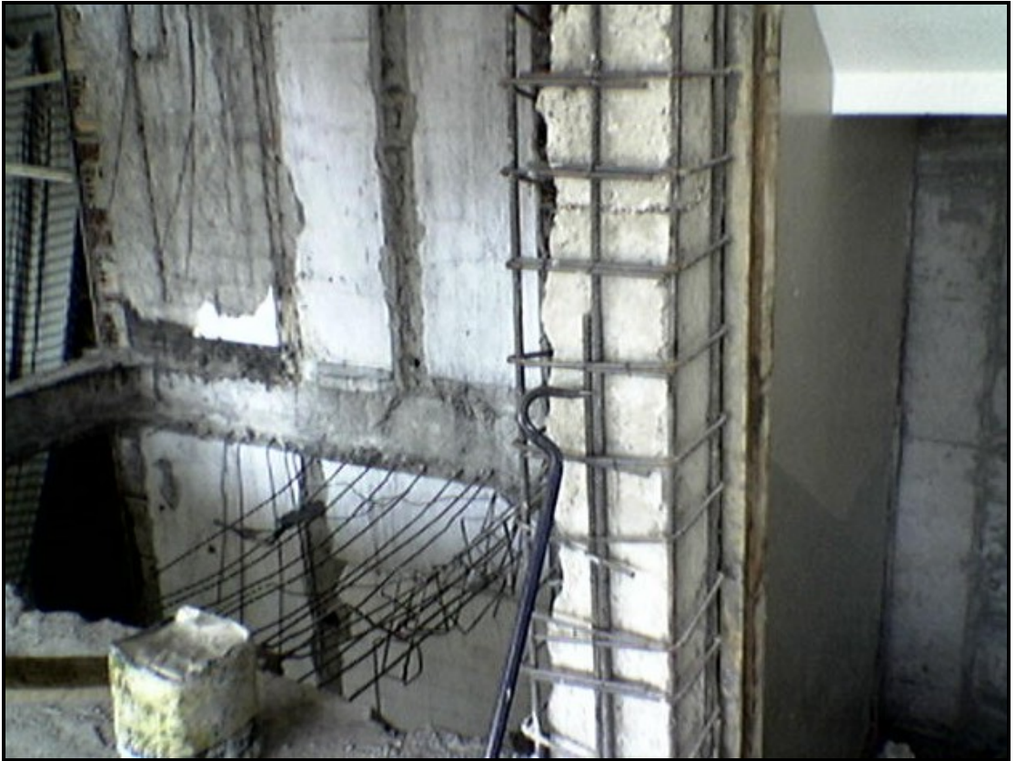
Figure 6.4. A Rehabilitated Column by using Jacketing Method (Courtesy of Rehber Yapı Denetim San. ve Tic. A.Ş.)
