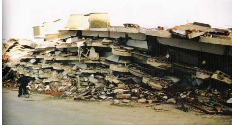
Figure 3.30. Damage due to the hollow-tile floor slab (Source: Çiftçi, 1999)
