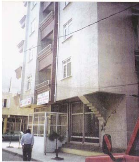
Figure 3.27. Damage due to the gusset on columns (Source: Çiftçi, 1999)
