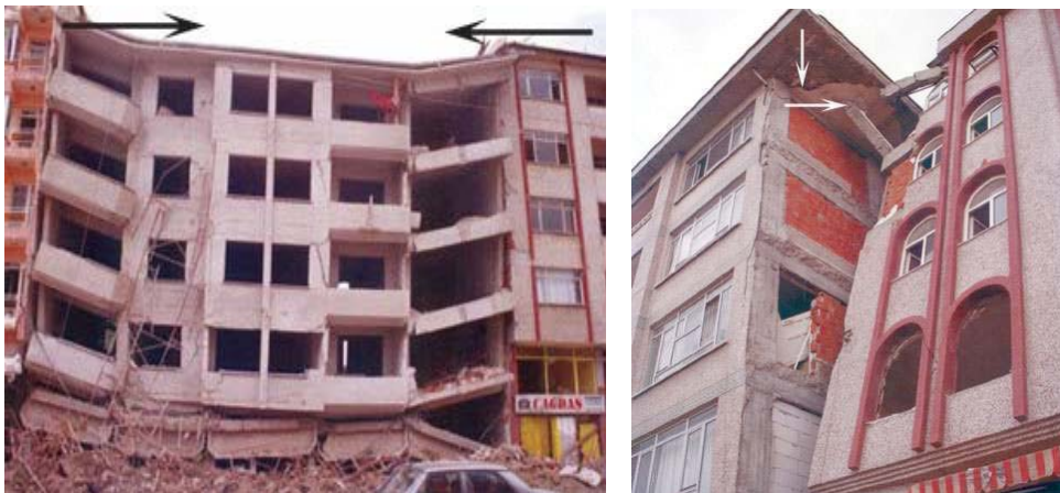
Figure 3.31. Pounding due to the torsion between adjacent buildings (Source: İstanbul Büyükşehir Belediyesi Devlet Arsivi, 1999)
