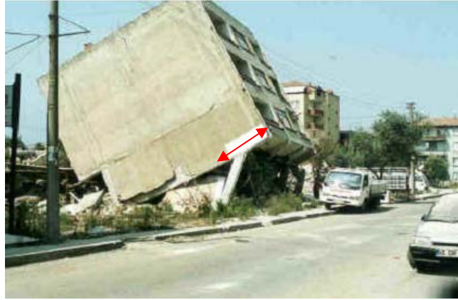
Figure 3.20. Damage due to the heavy cantilevers (Source: Darılmaz, 1999)
