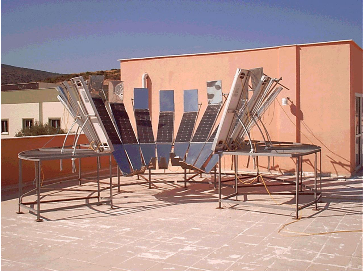
Figure 4.2 Omega Type Solar Charge Station on Classroom's Building rooftop.
