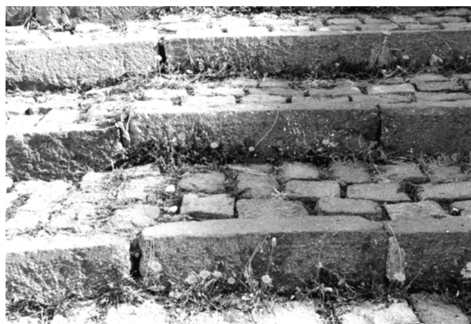
Figure 5. 61: Steps on 334 th street (April 2001)
