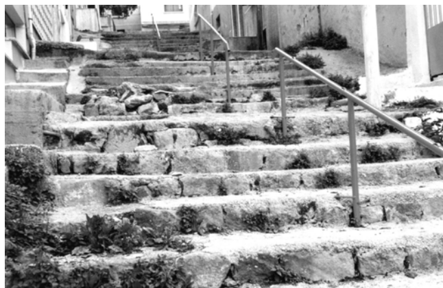
Figure 5. 71: Handrails that are broken up at landings on 309 th street (September 2001)
