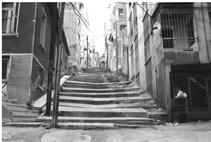
Figure 5. 64: Damaged concrete steps on 340 th street (September 2000)
