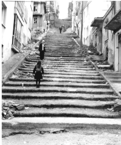
Figure 5. 104: Damaged concrete steps (September 2000)
