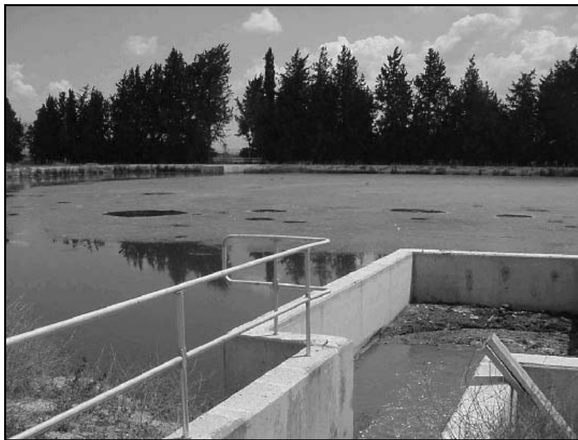
Figure 5.7 Useless wastewaters in Lefkoşa Haspolat Treatment Plant
