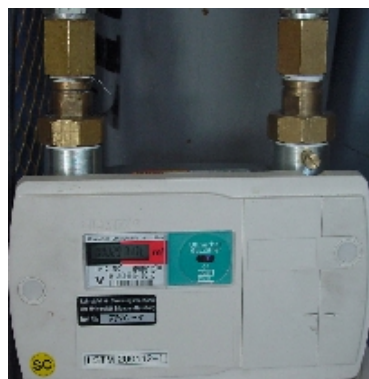
Figure 4.7. Adaptive 2000 domestic gas meter
