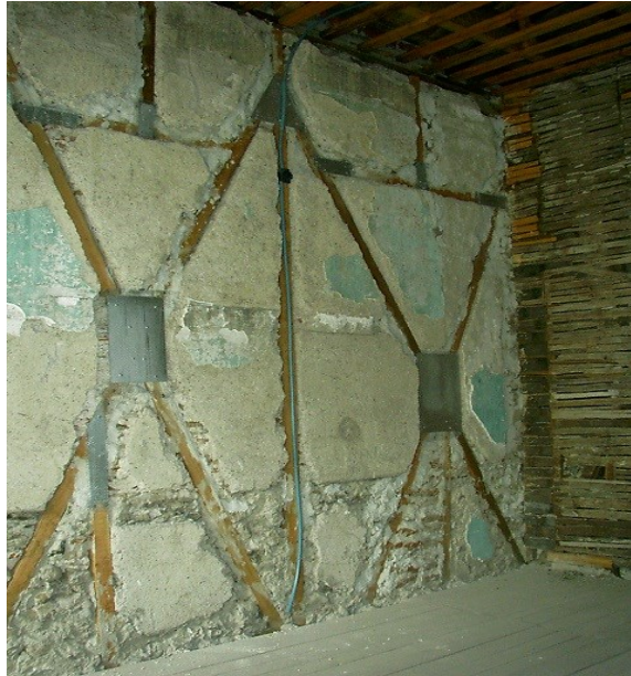
Figure 3.7. The traditional himiş system and structure of partition walls (Source: Archives of Architectural Restoration Department IZTECH)
