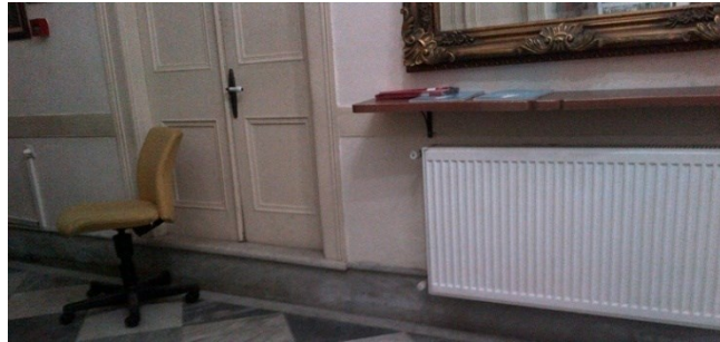
Figure 3.18. A hot water radiator in the building
