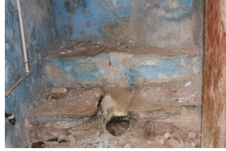
Figure 37. A view of toilet pan in the toilet (B11)
