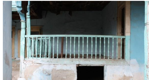
Figure 48. A view of the hall (G07) and the entrance of storage (B12)
