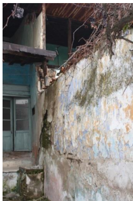
Figure 139. A view of the additional walls on the first floor and courtyard
