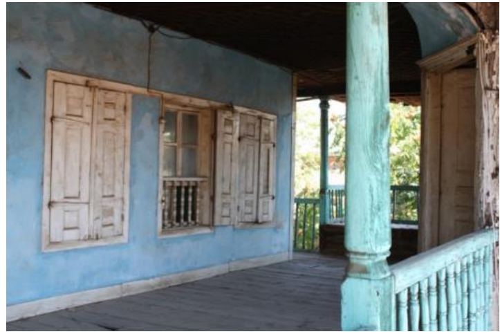
Figure 62. A view of the hall- F01, the window system of F08 and the entrance door of F11
