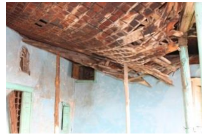
Figure 150. The collapse of roof and ceiling
