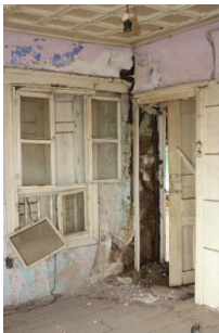
Figure 148. The damages in F11 (room)
