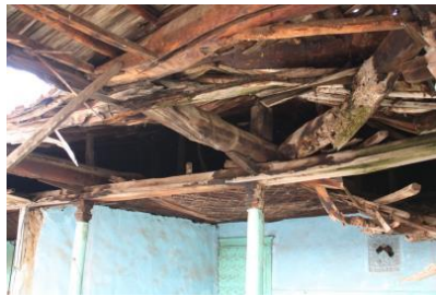
Figure 149. The collapse of roof and ceiling
