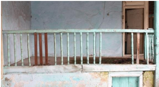
Figure 47. A view of the hall (G07) and the entrance of stable (B10)
