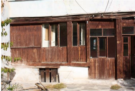
Figure 142. A view of the additional panes on ground floor
