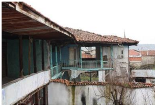
Figure 12. A view of main building from F02 (room) on the western corner
