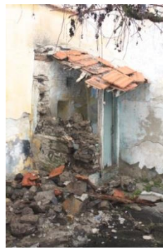
Figure 114. A view of the toilet in the courtyard unit- 1 on the plot 2
