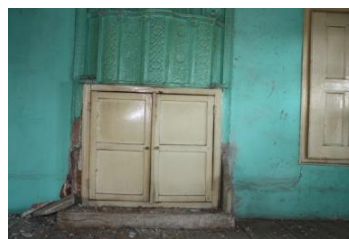
Figure 89. A view of the fireplace and the shutter of gusulhane in F08- room
