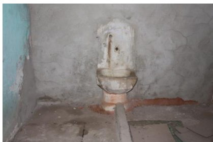
Figure 53. A view of the floor and the wash basin in bath- G10
