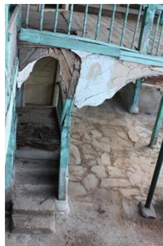
Figure 50. A view of entrance of the hall (G07) and entrance of room (G08)
