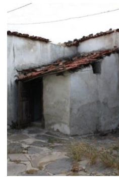
Figure 115. A view of the toilet in the courtyard unit- 2 on the plot 2
