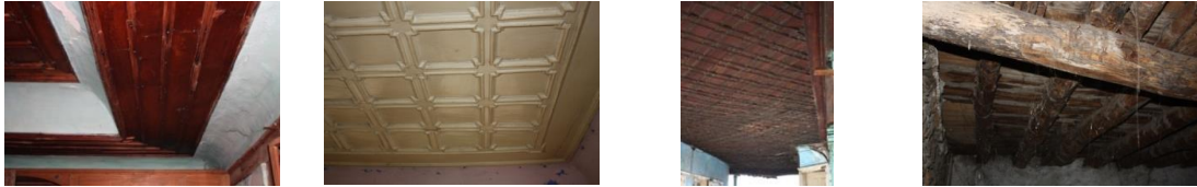
a) F02-room b) F11-room c) F01-hall d) B06-storage Figure 129. Views of the ceilings in the main building a) F02-room, b) F11-room, c) F01-hall, d) B06-storage
