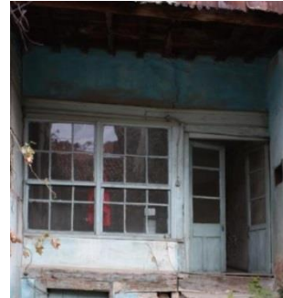
Figure 143. A view of the additional panes on ground floor
