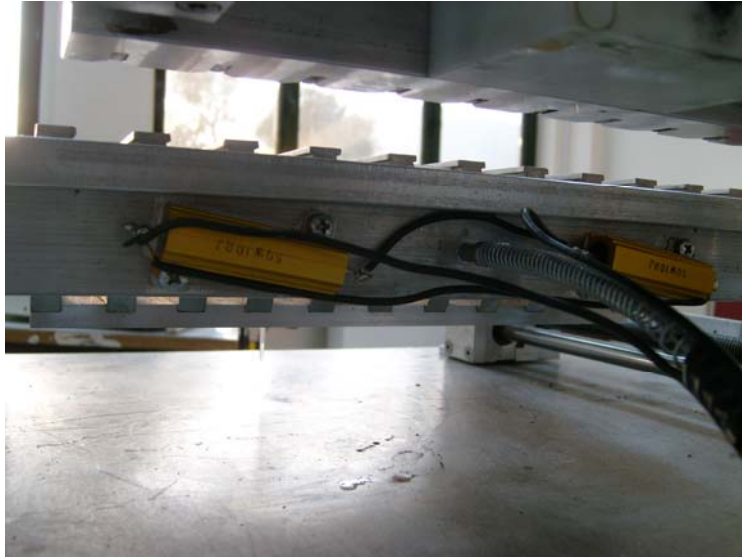
Figure C.8. Heater block, resistances and the thermocouple.
