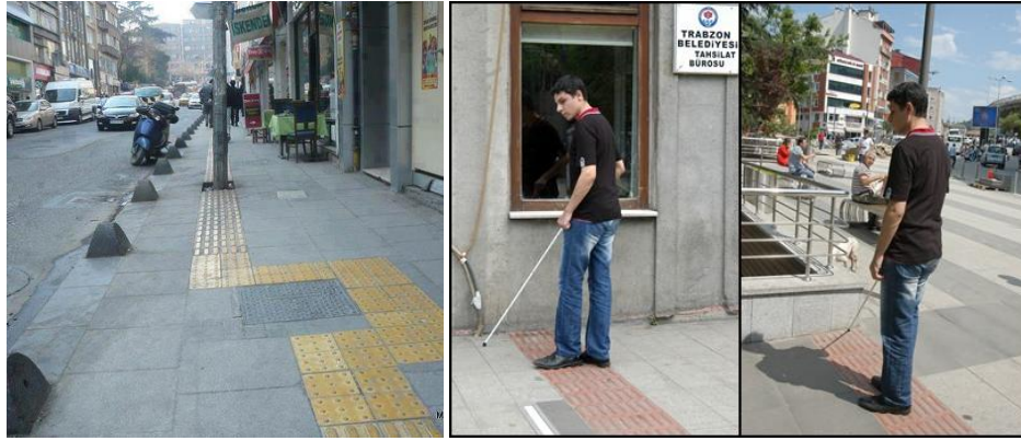
Figure 15. Some Faulty Implementations of Tactile Paving Stones in Turkey. (Source: http://www.kanalben.com/haber/7399/bu-kaldirim-engellilere-engel-oluyor.html and http://www.cumhuriyet.com.tr/?hn=343280 )
