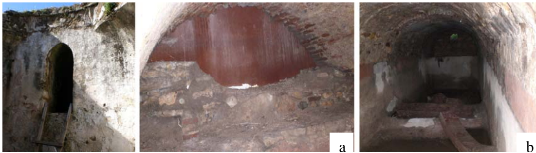
Figure 9. The window openings to the water reservoir (a) and the water reservoir (b)
