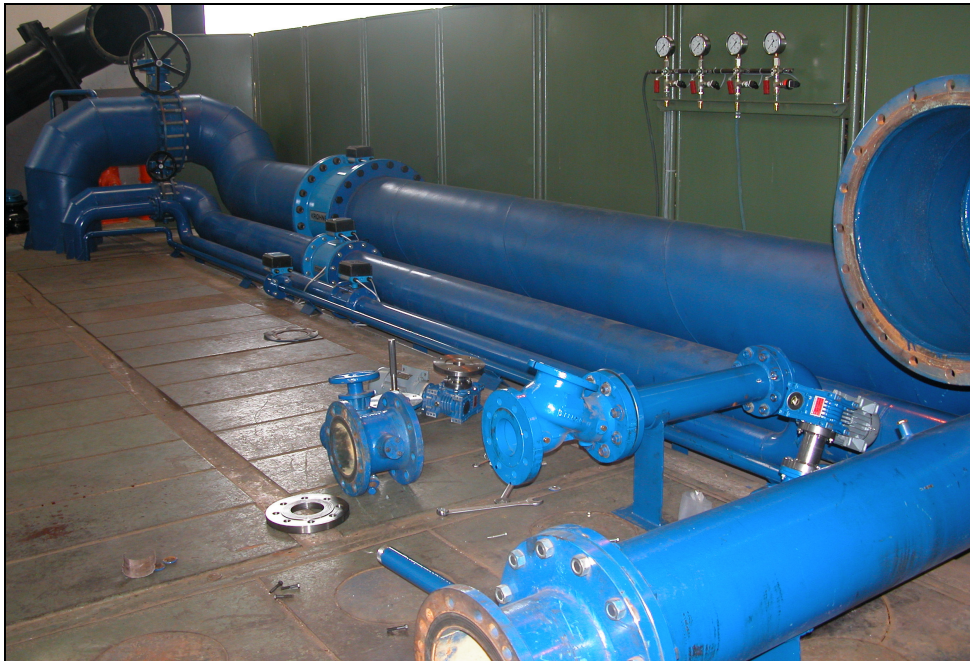
Figure 3.2. The flow meters, pressure transmitters, and the linearly controlled valves in the test process.
