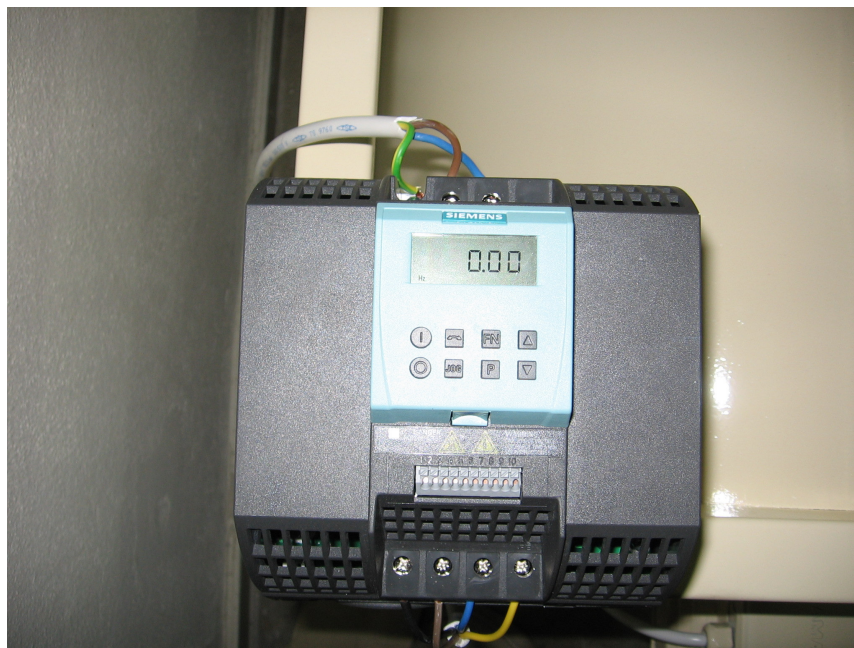
Figure 5.8. The frequency controller of the fan
