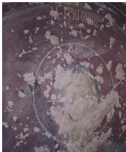
Figure 5.38. Loss of plaster and painting layer due to dampness in the painting no:4 on the main apse of the church
